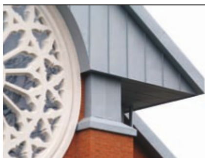
Project: St Georges Church, Catford Architect: Thomas Ford & Partners Installer: Metalex Traditional Metal Roofing Ltd
