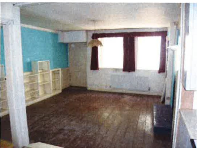
Overhaul and repair existing timber sash windows and panel door. Strip, stain and polish existing floorboards.
