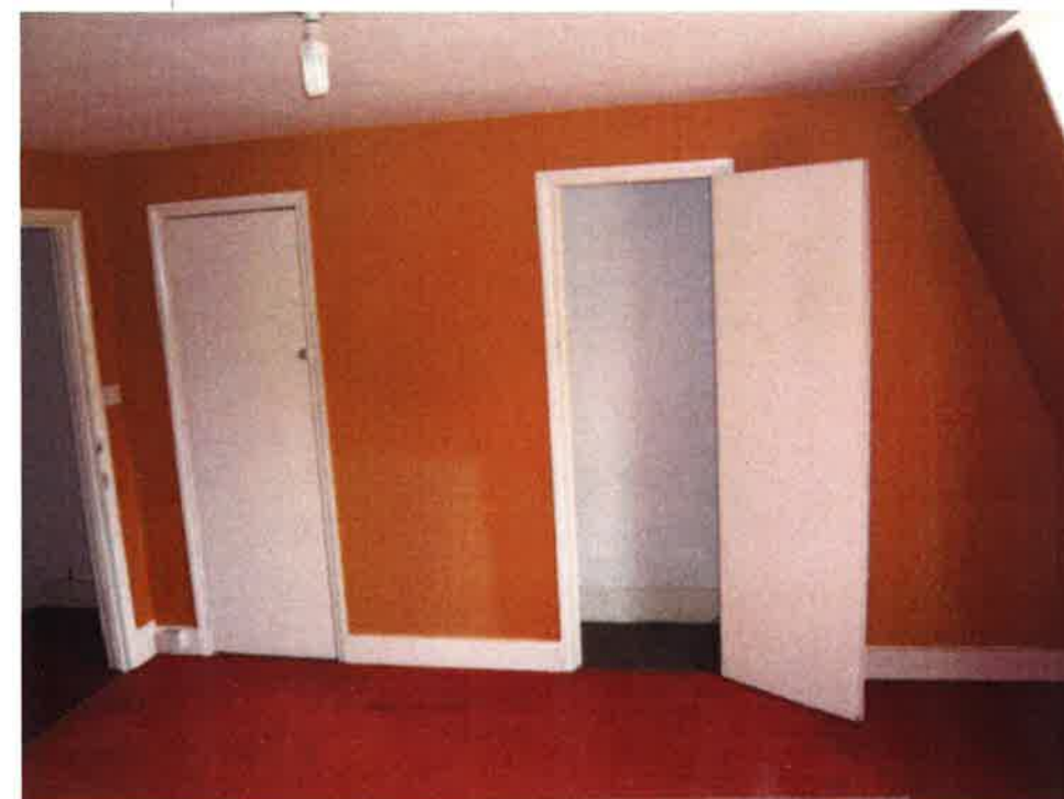
Remove new stud wall and doors and form new studwork wall to form bedroom and shower.
