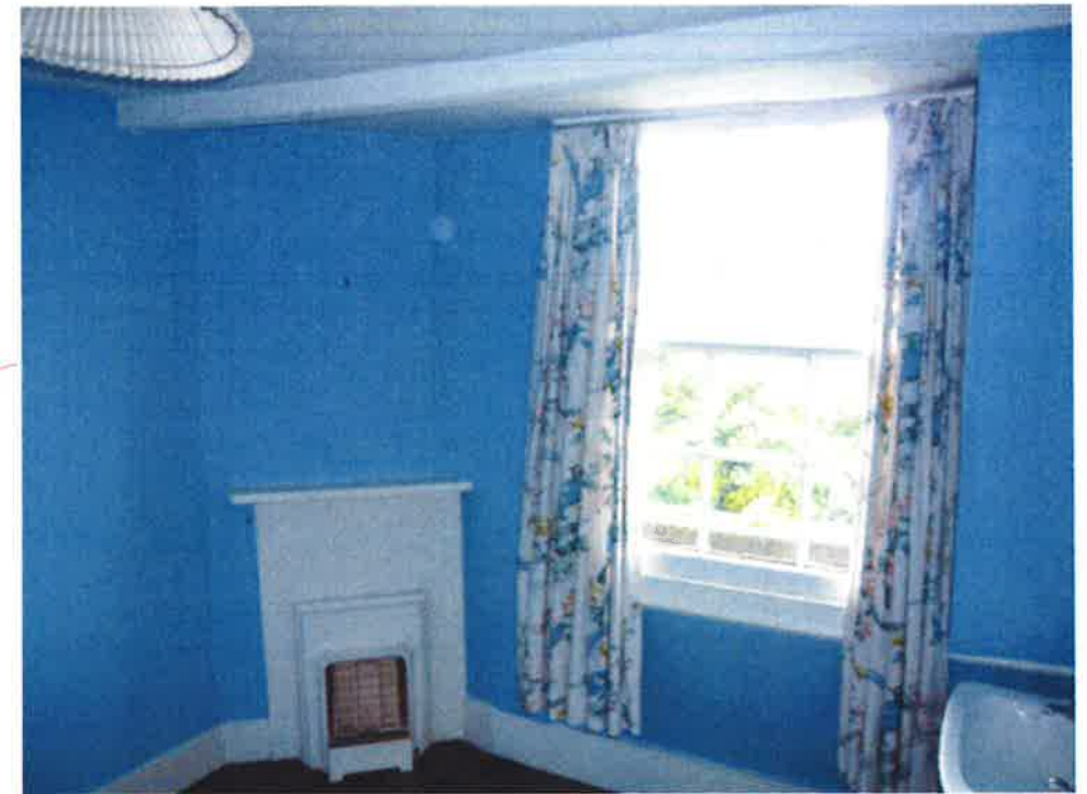
Overhaul and repair sash window. Retain fireplace surround and remove electric heater. Re-instate fireplace and hearth.
