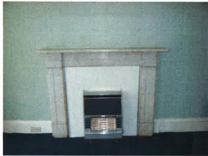
Existing fireplace surround to be retained. The fireplace and hearth to be reinstated.
