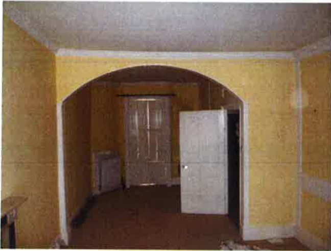
Retain, strip and repair; wooden wall panelling, sash windows and window shutters.
