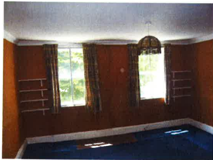
Overhaul and repair sash windows. Retain skirting and floorboards. Existing ceiling and cornice to be retained and repaired from water damage.
