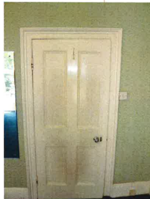
Strip and repaint timber door. Retain skirting and architrave. Remove cupb. door and retain door opening with architrave.
