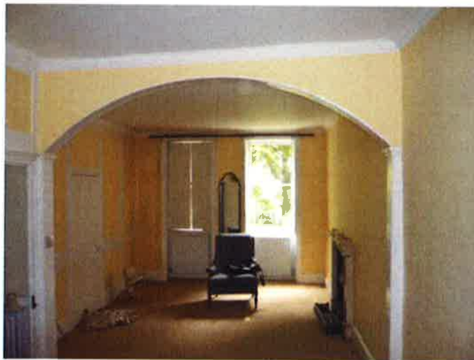
Retain, strip and repair; wooden wall panelling, sash windows and window shutters.
