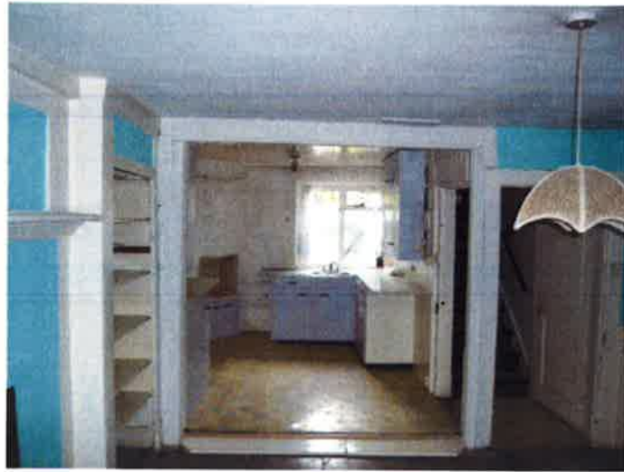
Remove lino, stain and polish existing floorboards. Hack off existing plaster, 1m from floor level, to install damp proofing and repair with lime plaster where applicable
