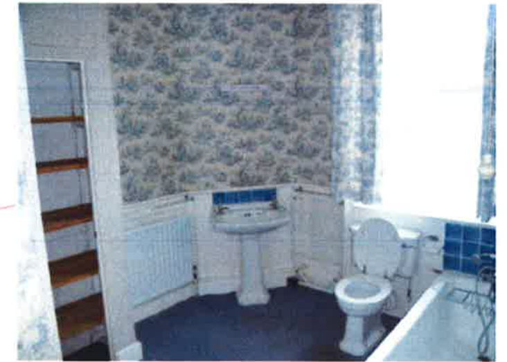
Overhaul and repair sash window. Repair and retain cornice. New bathroom stud wall partition shall have moulded plaster cornice and timber skirting to match the existing.
