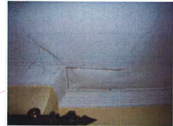
Retain and repair areas of water damaged lath and plaster ceiling and cornice.
