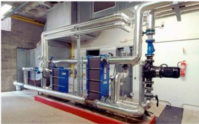
Figure 12: Example of prefabricated plate heat exchanger installation
