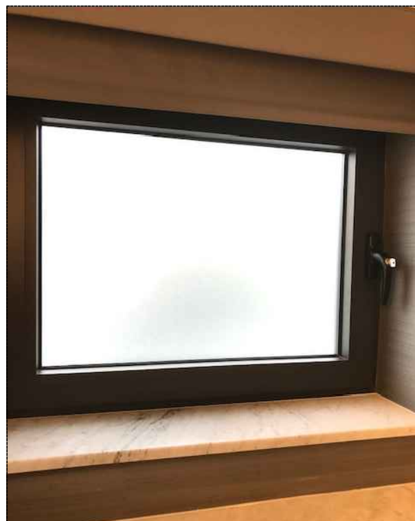
BOTTOM HUNG FROSTED GLASS WINDOW TO SECOND FLOOR BATHROOM. CLOSE POSITION.
