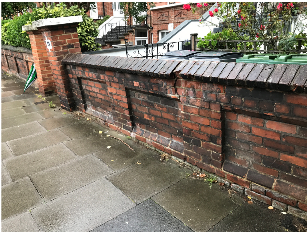
Section of wall showing further cracking damage and brickwork decay and a comparison of the two entrance piers shows the closest pier leaning over into the street.
