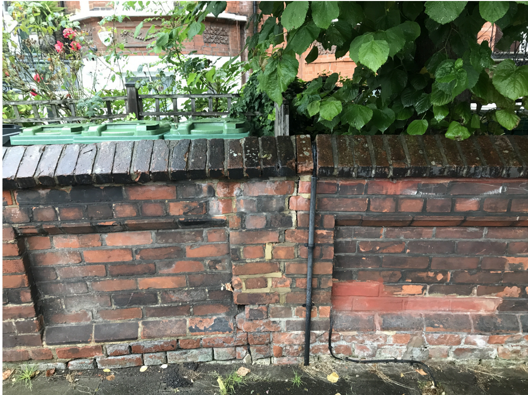
Section of wall showing cracking damage and brickwork decay.
