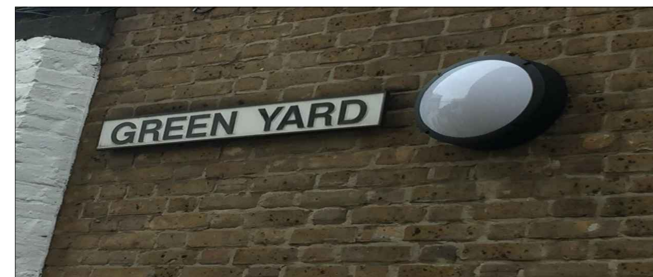
H - NIGHT LIGHTS WITHIN GREEN YARD ARE CLAIMED TO BE BRIGHT AT NIGHT AND SHINE TOWARDS WREN STREET. THERE ARE 14 OF THESE SET AT REGULAR SPACES THROUGH THE PERIMETER OF GREEN YARD. LIGHTING TO BE REPLACED WITH SENSOR CONTROLLED LIGHT FITTINGS.
