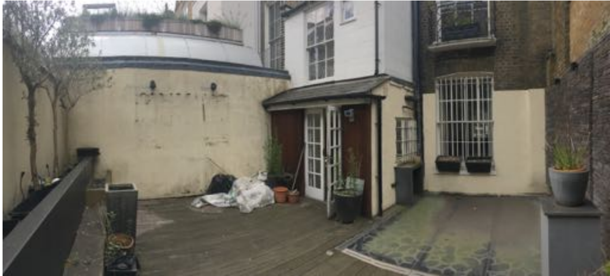
Photograph taken in July 2017 showing the existing space at the rear of no. 17 John Street which is deteriorated and unused by the occupants.
