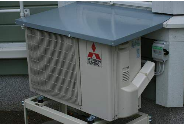
Figure 11: Outdoor unit of an ASHP
