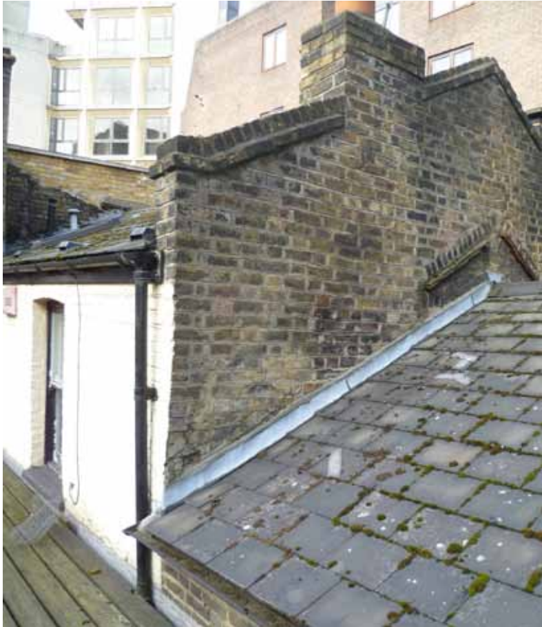
Existing Site Photos : view of the existing roof and rear of the site
