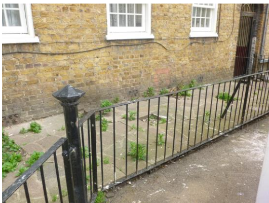
Existing raised paved areas and low railing to be removed and new raised planting beds to be created.
