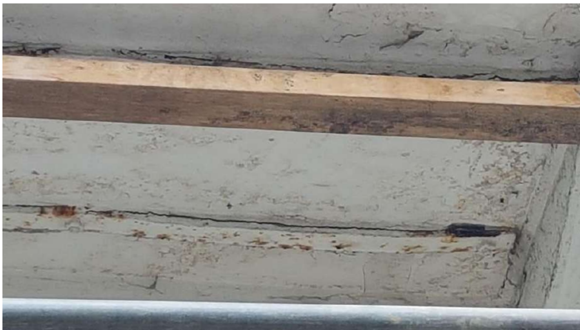
View indicating steel/iron support straps – note corrosion
