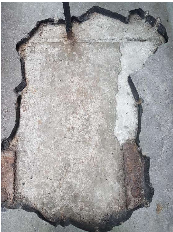
View of steel straps from top, require replacement and renewal to detail
