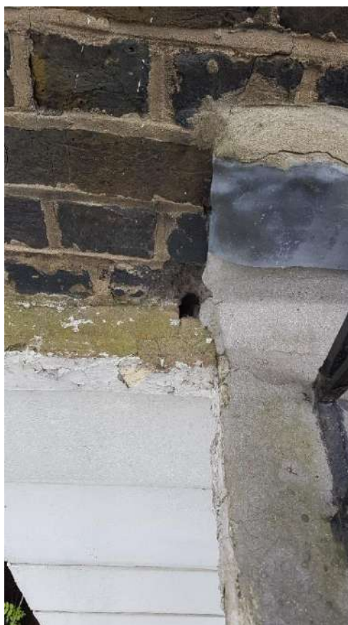
View showing small hole in wall
