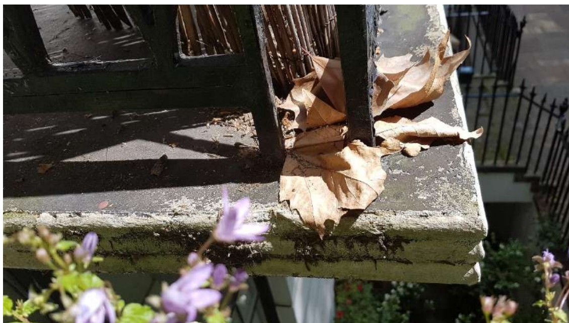
Neighbouring property with no screed or asphalt on surface of balcony stone.
