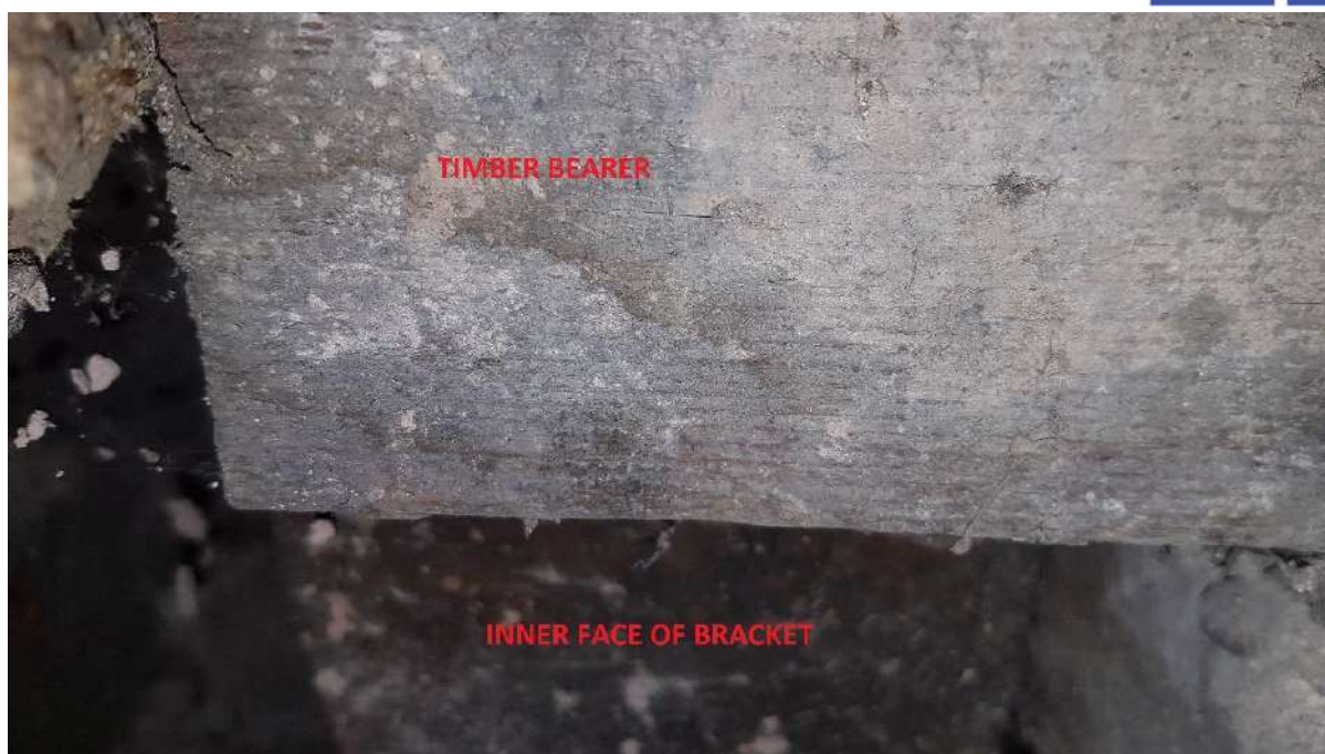
View of rear of bracket and timber bearer from opposite end of brick pier.
