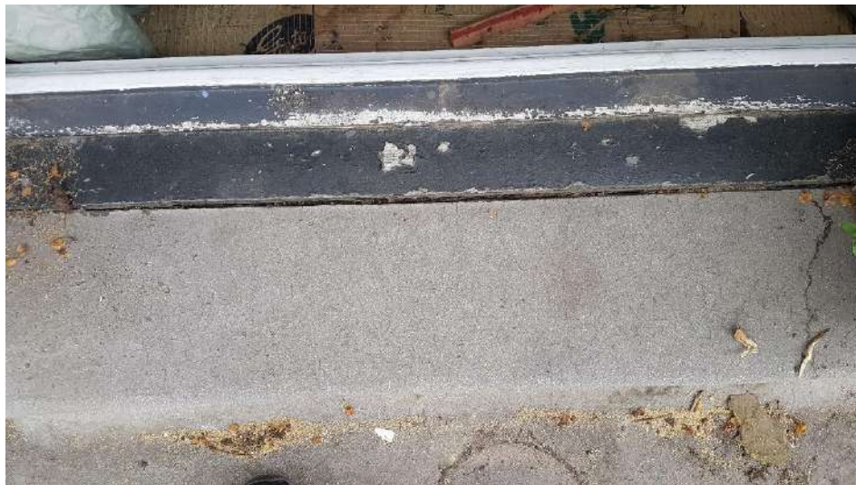
View showing gap between back of asphalt and window frame
