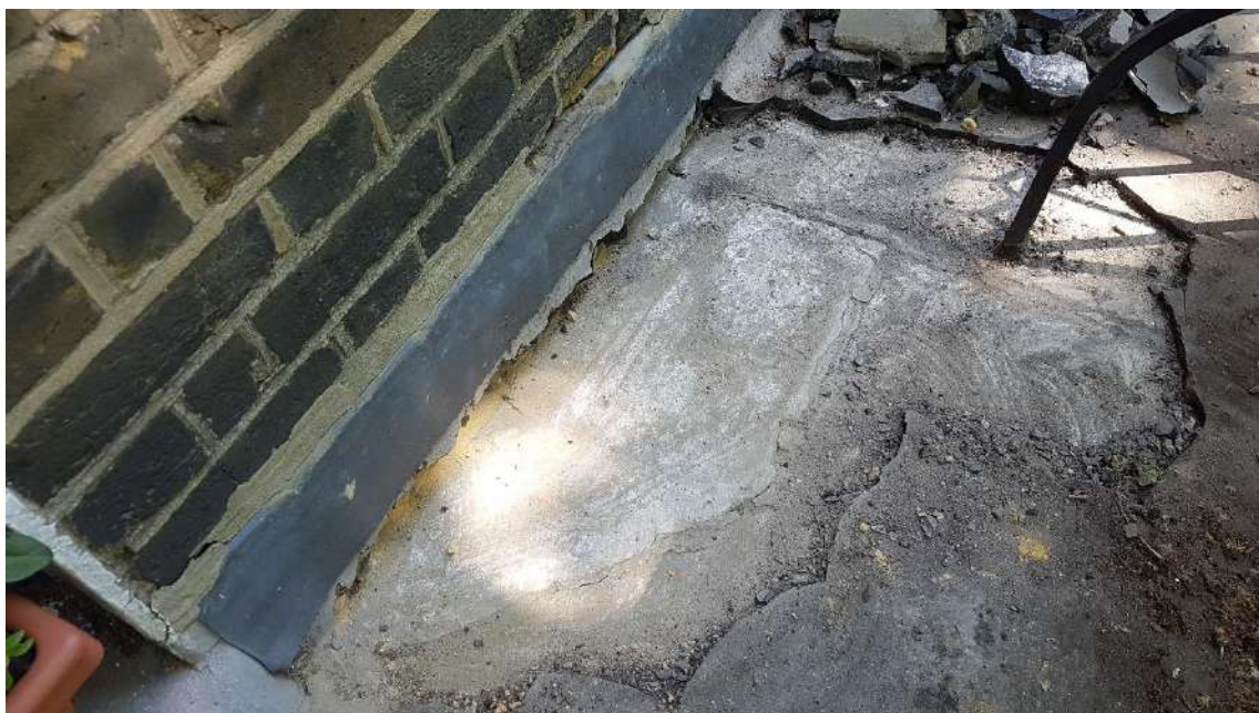
Western Joint - Detail of differing screeds. Note the screed that tapers out to the main wall.
