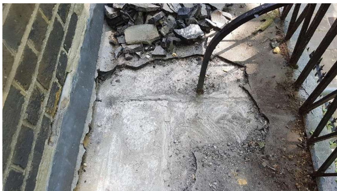
Removal from the Western Joint - Asphalt approximate 20/25mm thick on cementitious repair
