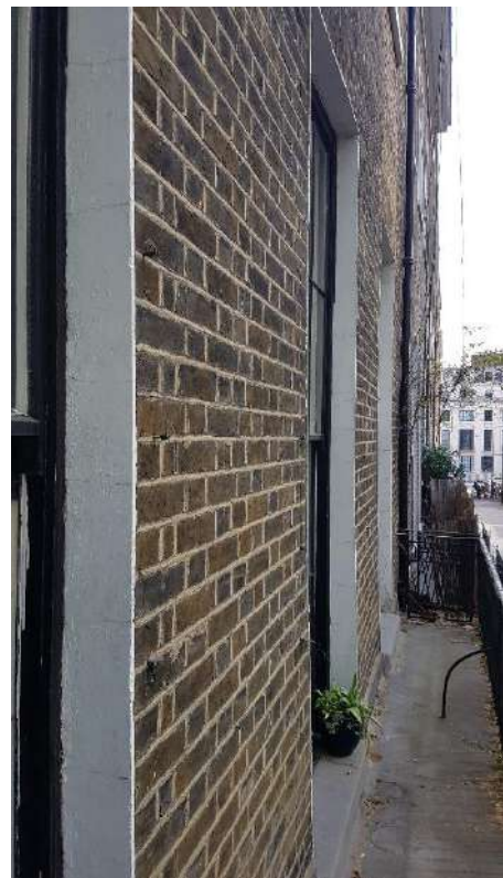
Window reveal render cracking
