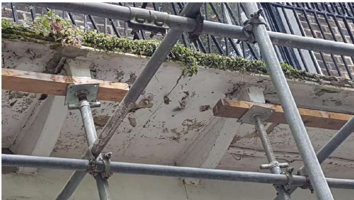
Vegetation on edge of balcony, balcony stone joint shown.
