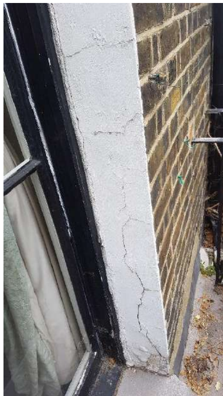
Window reveal render cracking
