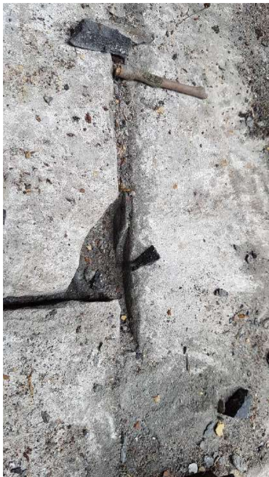
Western Joint - Corner of screed removed with the inverted T shown between the joint.
