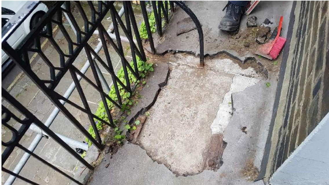
Removal from the Eastern Joint over the front door, showing the reinforcing steel and fixings, Asphalt 50-60 mm thick
