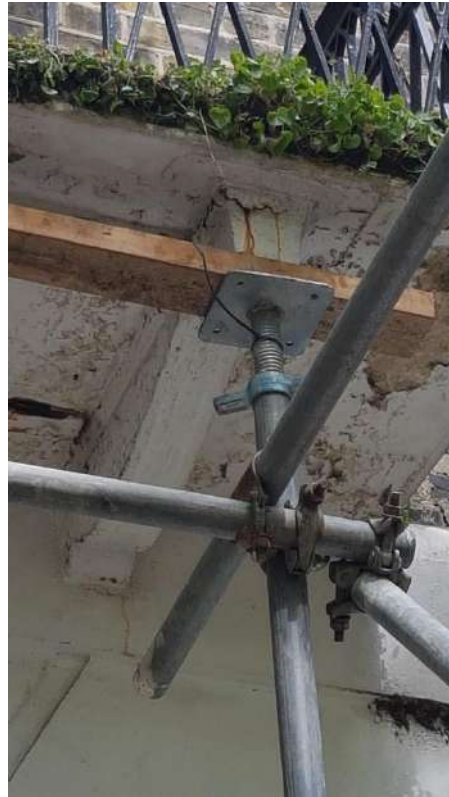
Bracket surface corrosion
