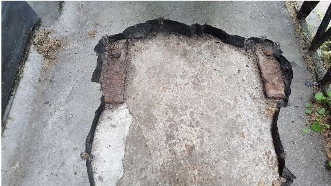
View of steel straps from top require replacement and renewal to detail
