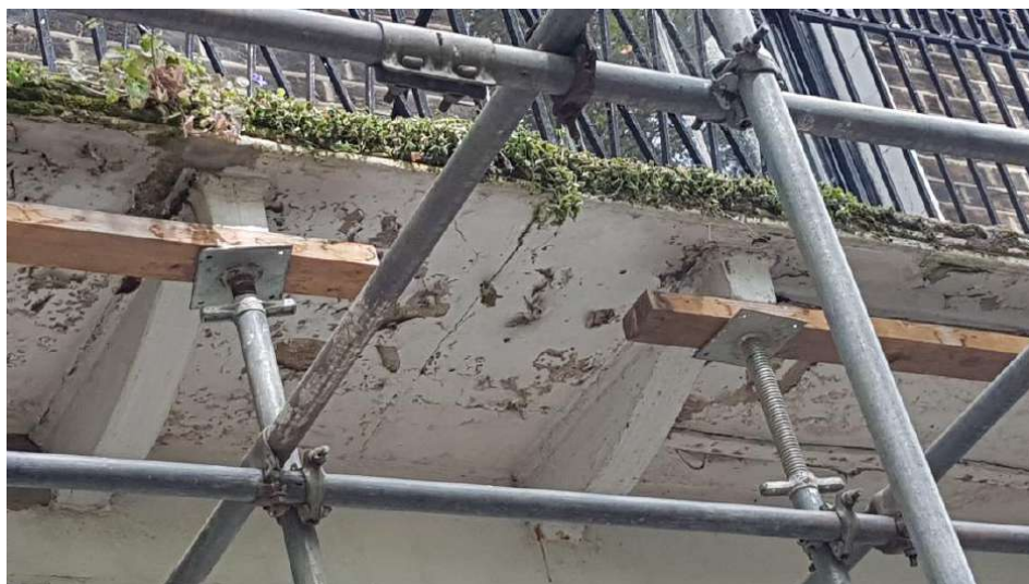
Flaking and missing paintwork – stone abutment shown between brackets
