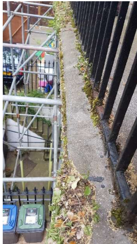
Vegetation on edge of balcony and collecting around bottom of the balustrade, trapping water
