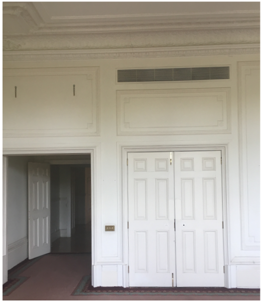
A/C vents to be removed and replaced with new plaster mouldings to match existing
