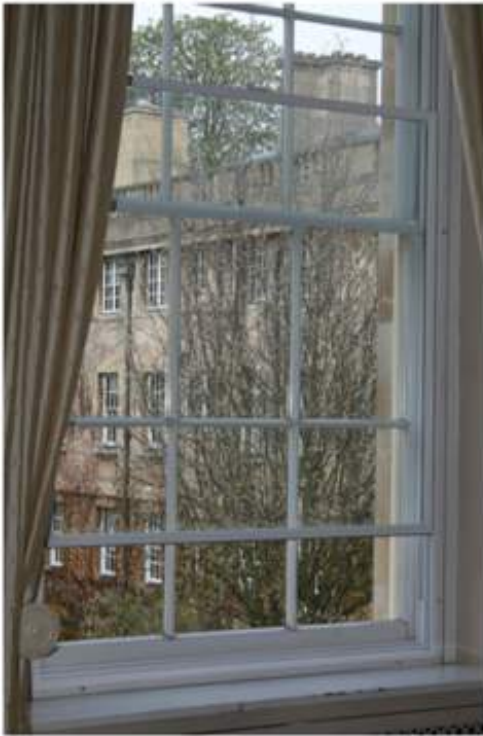
Internal View - N.B. intrusion into reveal and compromise of architrave details, difficulty of access to open outer window
