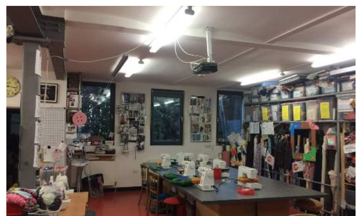
Interior view of existing ground floor workshop looking towards the rear windows and yard - proposed to form openings to the new extension.
