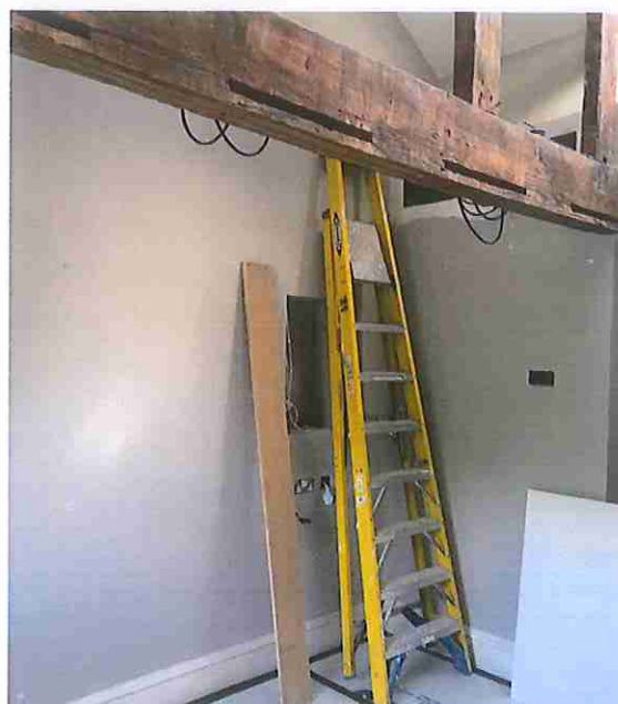
Photograph of modern plasterboard lining installed in front of chimney breast. To be removed. New ceilings to be installed below timber roof structure.
