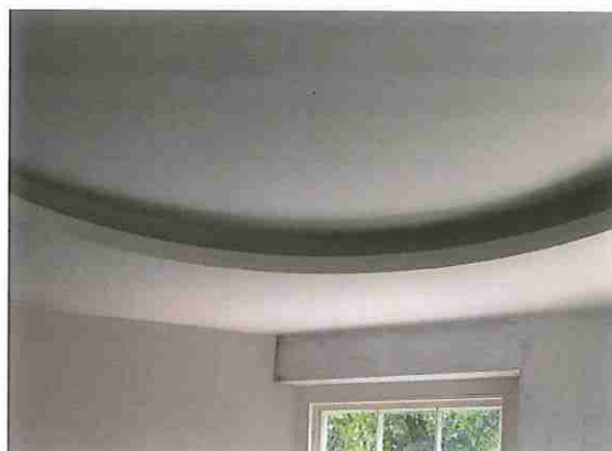
Photograph of as installed modern ceiling arrangement in rear bay. Simple flat ceiling arrangement to be installed in its place.
