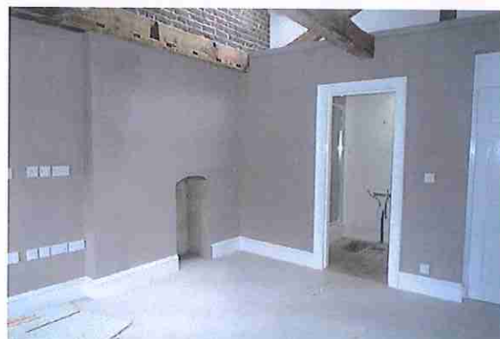
Images taken within the third floor prior to the 2014 application. Note the open ceilings, modern plasterboard wall finishes and ceiling linings and a number of rooflights.
