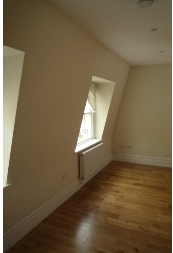
Image taken within the second floor flat prior to the 2014 application. Note modern finishes, recessed light fittings and surface mounted radiators.
