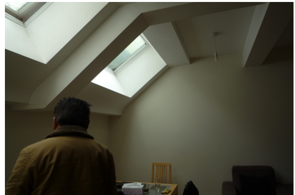
Image taken within the first floor flat prior to the 2014 application. Note the plasterboard bulkhead arrangement to conceal modern steel floor and roof structure.
