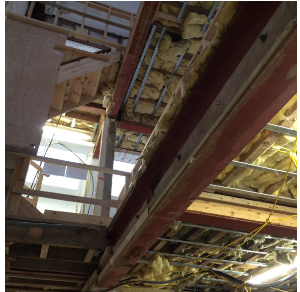
Image provided by the Contractor taken from the ground floor level looking up. Modern steel and timber joist arrangement with insulation infill.
