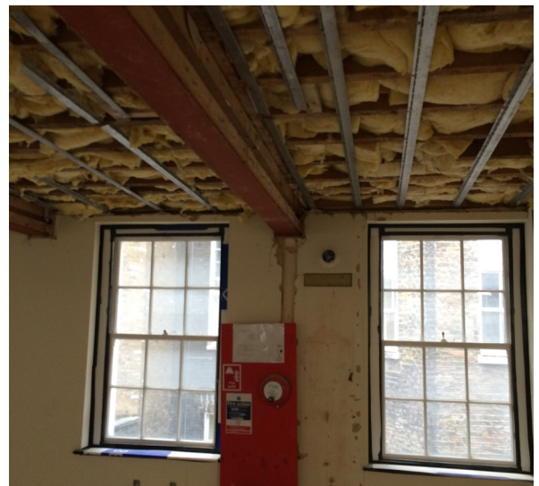
Image provided by the Contractor taken within the first floor level looking north towards the main house. Note the steel arrangement and relationship with the adjacent window openings.
