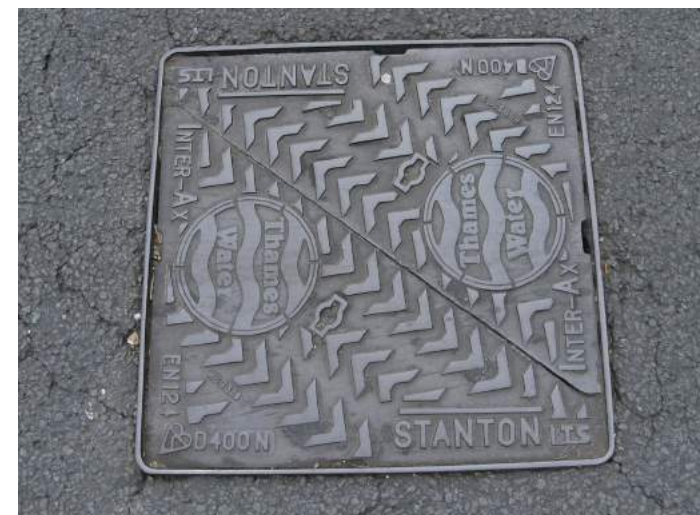
Figure 6.1d Thames Water access cover, Finchley road, London.
