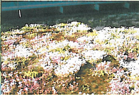
Moss growth due to standing water
