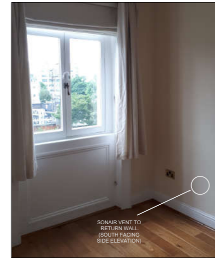
SONAIR VENT TO RETURN WALL (SOUTH FACING SIDE ELEVATION) SEE DRAWING P2229-PVE34-SE-P
