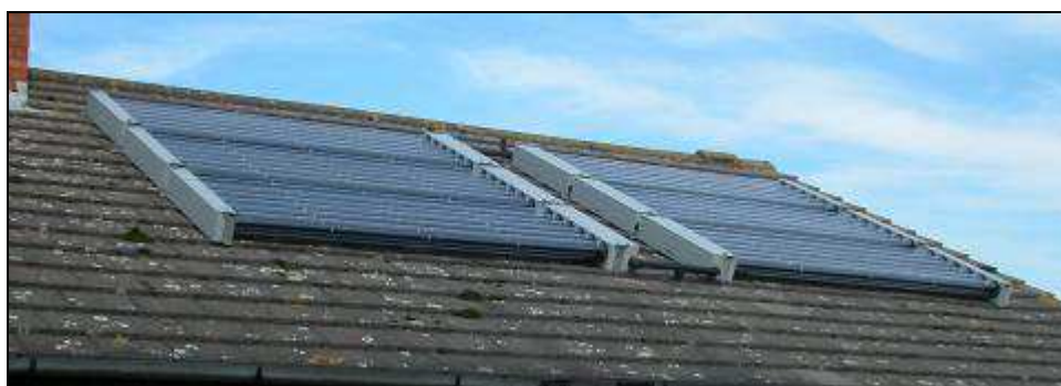
Figure 14: Evacuated Tube Solar Collectors
