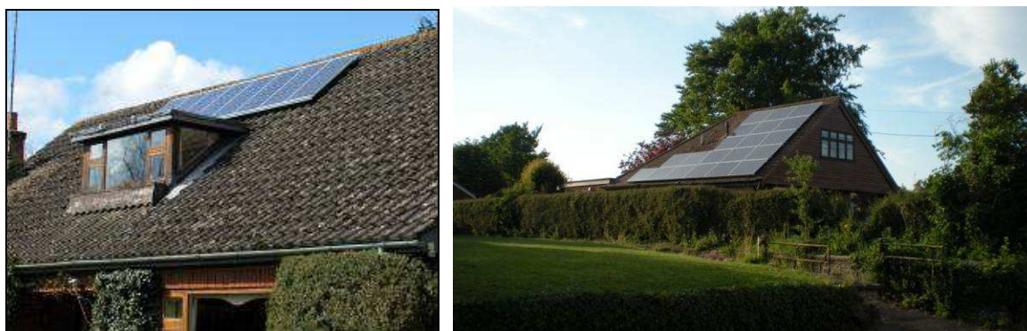
Figure 10: Standard PV panels installed on a houses in Berkshire and Oxfordshire
