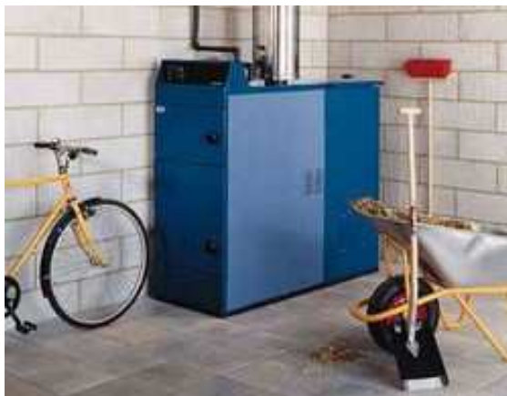
Figure 3: Standard domestic pellet boiler (Baxi)
