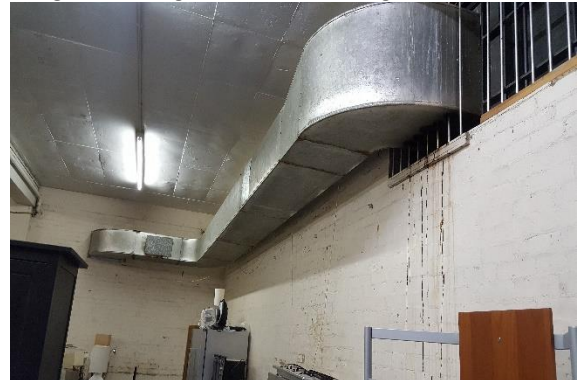
Image 4 – Existing internal plant equipment
