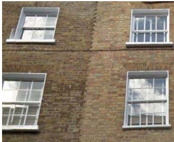
Figure 1: mismatched brickwork between 7 and 8 Sandwich Street
