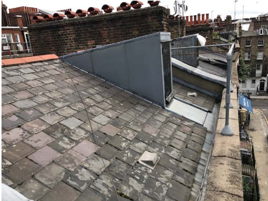
Figure 6: typical example of roof access dormer to similar neighboring buildings (6 Sandwich Street shown in the foreground)
