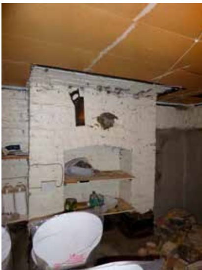
20. Blocked coal chute at basement level, room B02 (2016), DIA
