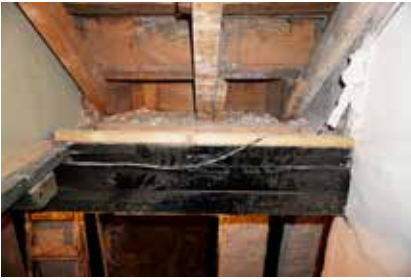
26. Original ground floor stair trimmer, now redundant due to the relocated position of the stair; (2017) DIA
