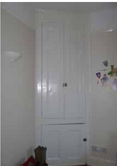
25. First floor corner cupboard possibly made out of re-used window shutters, room F03 (2016), DIA
