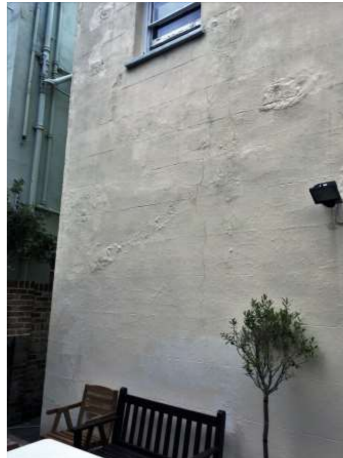
Plate 2: Spalling render on side elevation
