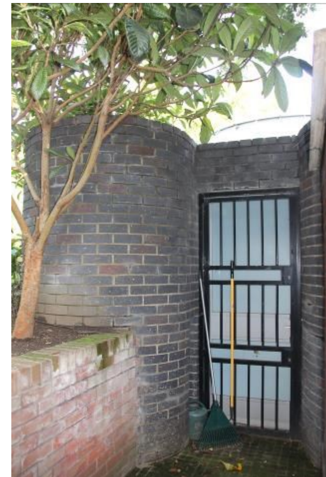
Figure 23: Original entrance to the pool now locked up and featuring altered wall details either side
