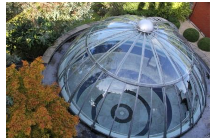
Figure 17: View of the pool showing loss of mound
