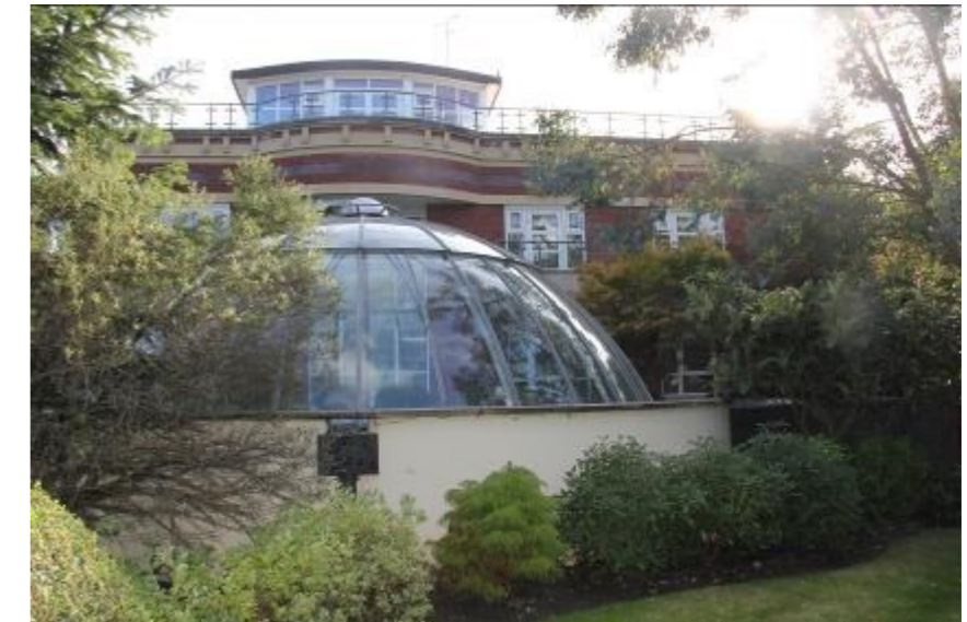
Figure 16: Note the loss of the original mound, and presence of harsh retaining wall and exposed down pipe with hopper
