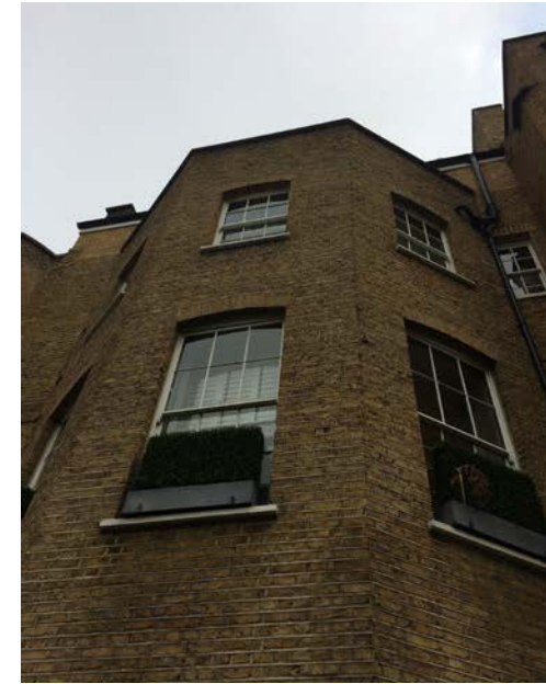
Photo of current state of the rear elevation of no. 34 following work in 2007
