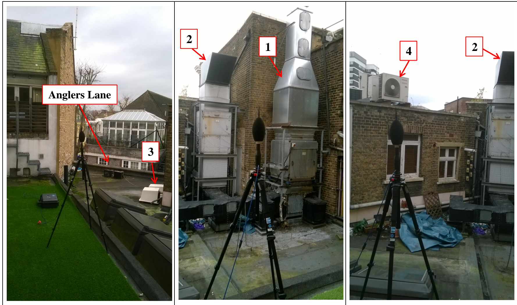
Figure 7.1: Photos of monitoring location 2 and plant units operating at the Site Surroundings
