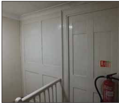
Photo 7: Wooden panelling and blocked door in No. 109 third floor / attic level, hallway
