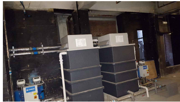
Photo of existing plant
