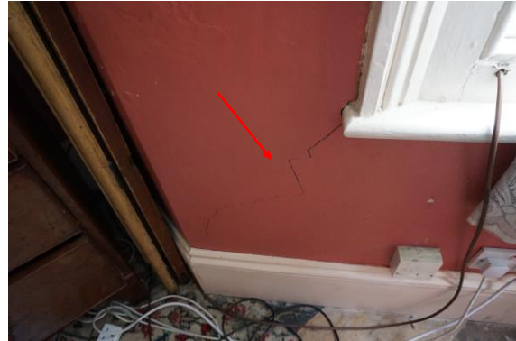
GF Front Bedroom – Diagonal Crack at Bay Junction
