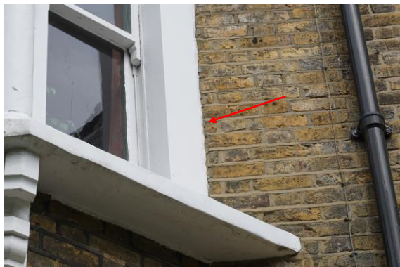
FF Bay – Separation at Junction to Main House
