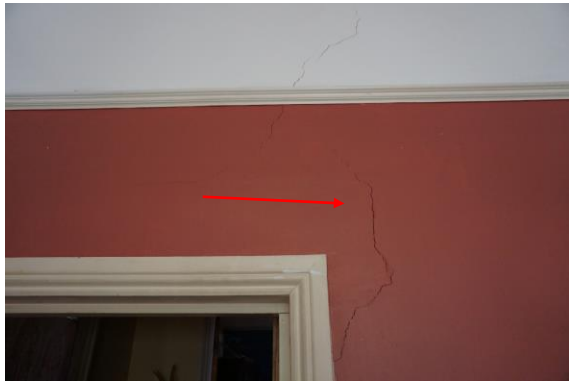
GF Front Bedroom – Vertical Crack Above Door to Lobby
