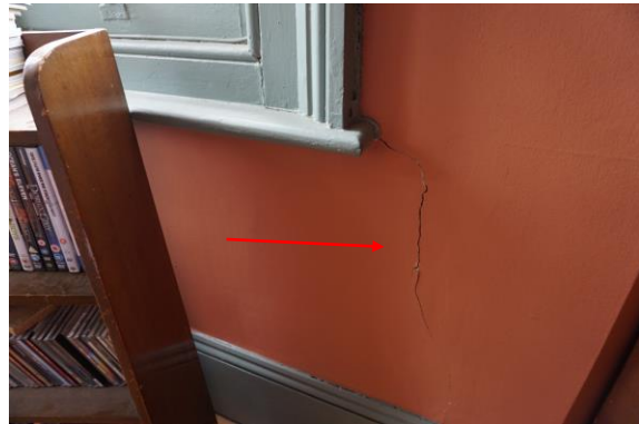
FF Front Bedroom – Diagonal Crack to Bay Junction
