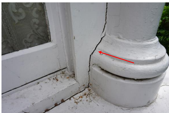
Front Bay – Stonework Separation
