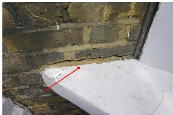
Front Bay – Separation of Sill from Main House
