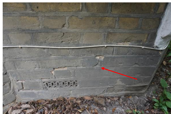
Front Bay – Stepped Cracking
