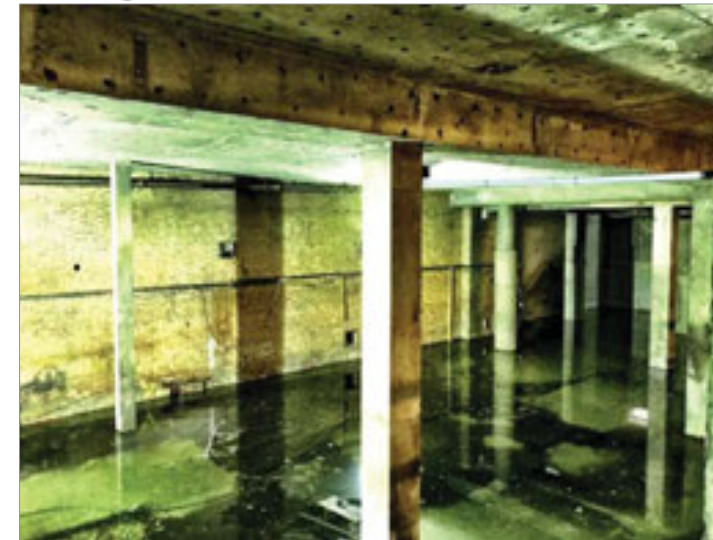
3.01 Retained Ground Floor slab and supporting beams and columns at the north of the site at high level basement.
