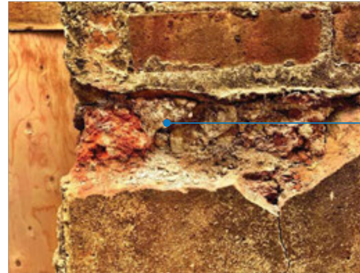
4.05 Snapped off stretcher bricks at the end of the wall. It would appear that the wall originally continued into the site to form a boundary wall between the two previous separate titles.
