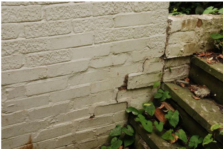
Photograph 7: Cracked brickwork to rear addition
