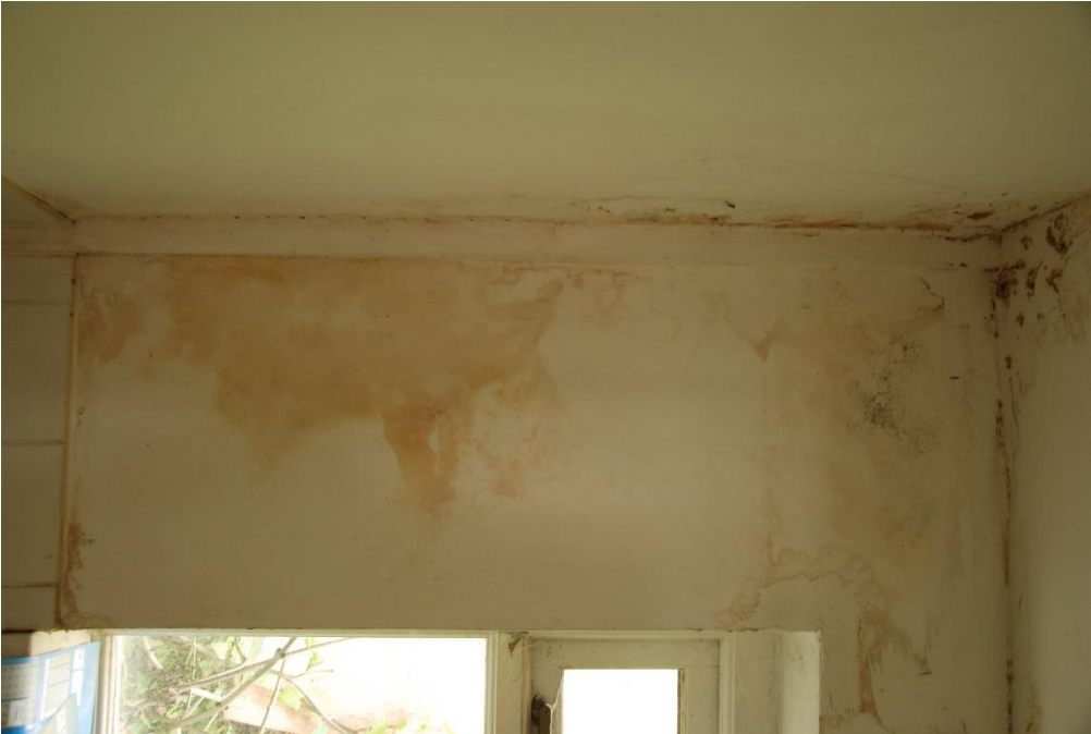
Photograph 21: Dampness to interior walls
