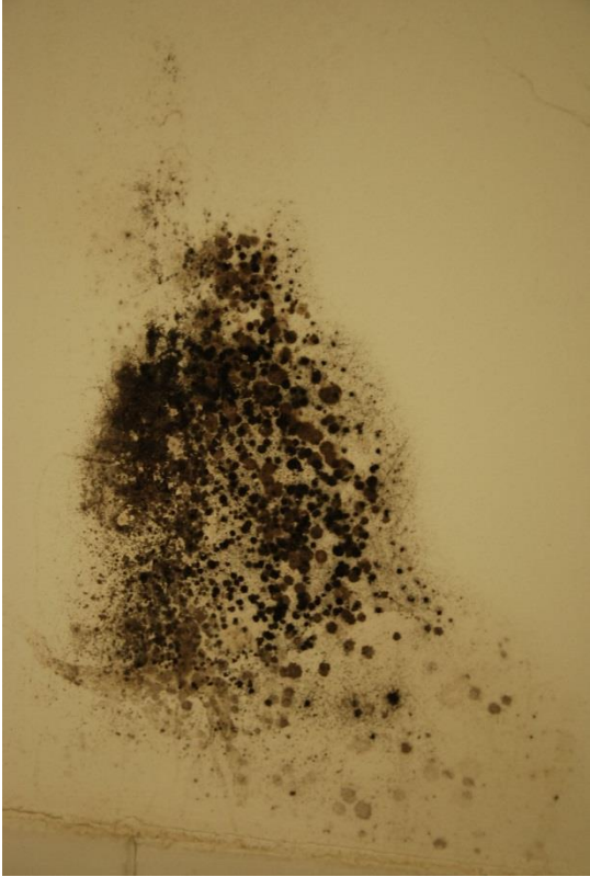
Photograph 19: Mould in interior
