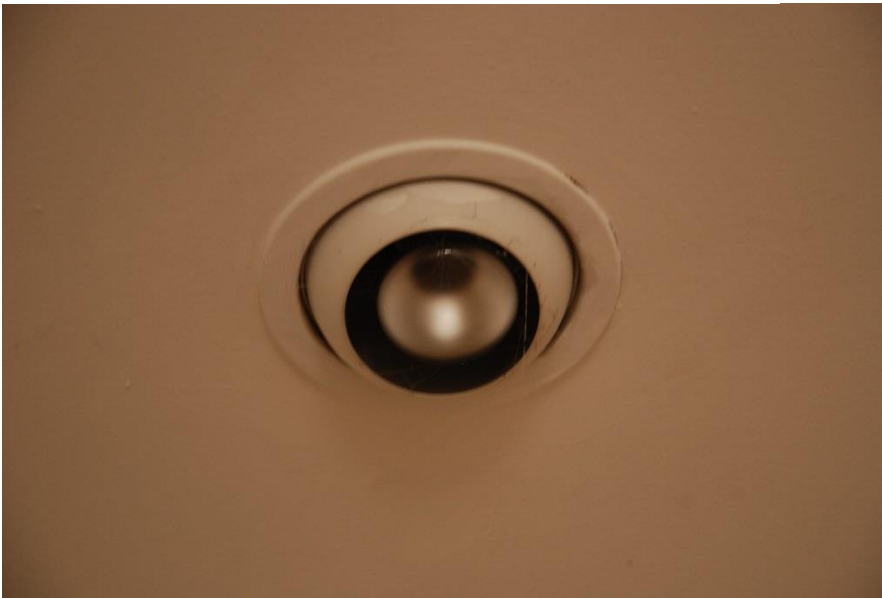
Photograph 27: Existing typical light fitting
