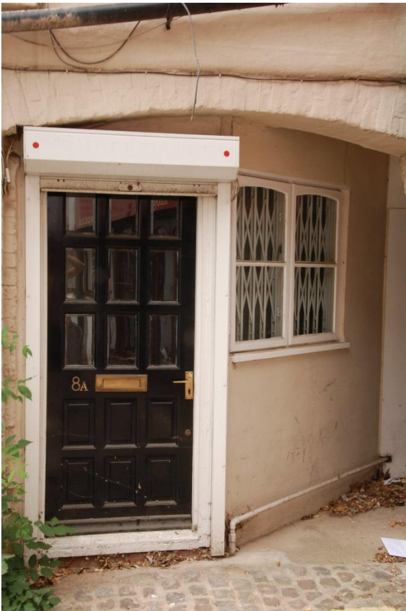
Photograph 10: Front door and security shutters
