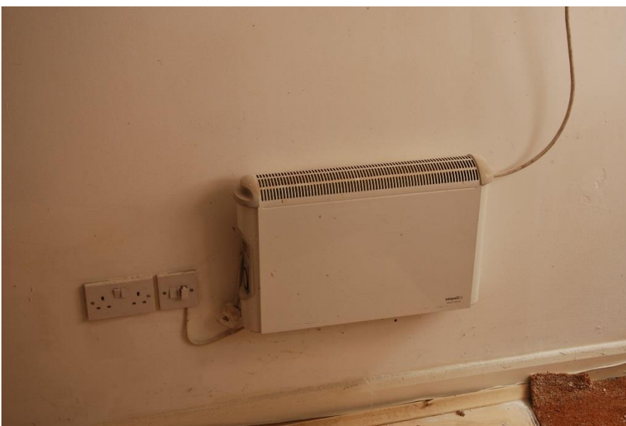
Photograph 28: Electric Dimplex heater
