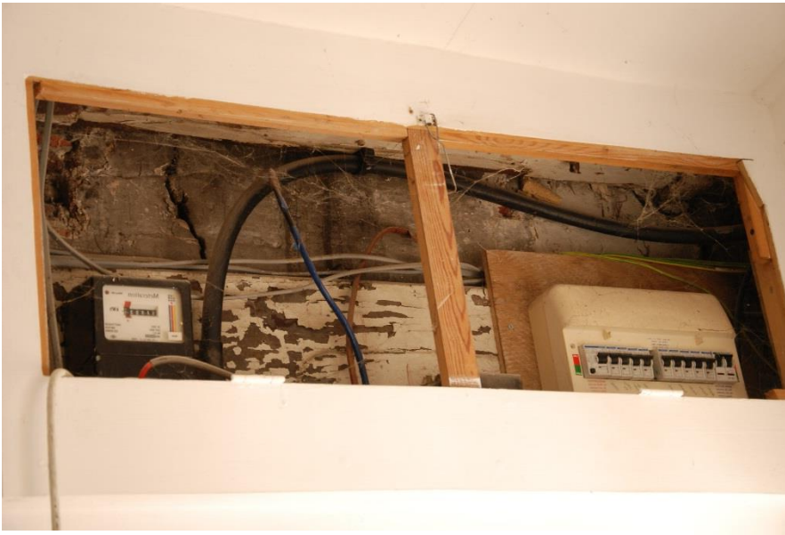
Photograph 26: Electric meter and fuse board
