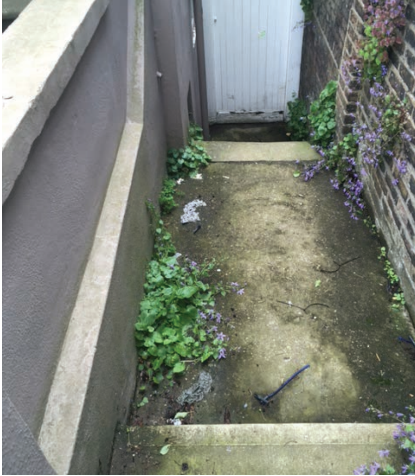
External side steps at 10 Provost Road - low grade rough concrete slab
