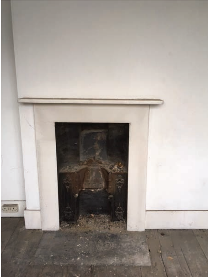
Second Floor Fireplace existing condition:, with crumbling inserts and low grade surrounds which are to be replaced with suitable period replacements
