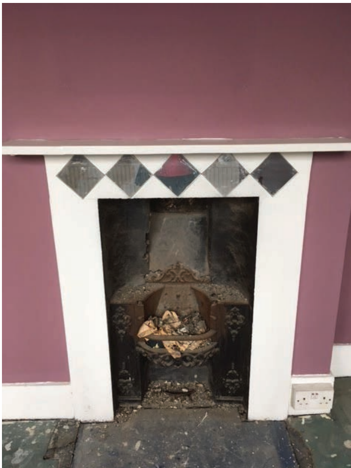
Second Floor Fireplace existing condition:, with crumbling inserts and low grade surrounds which are to be replaced with suitable period replacements
