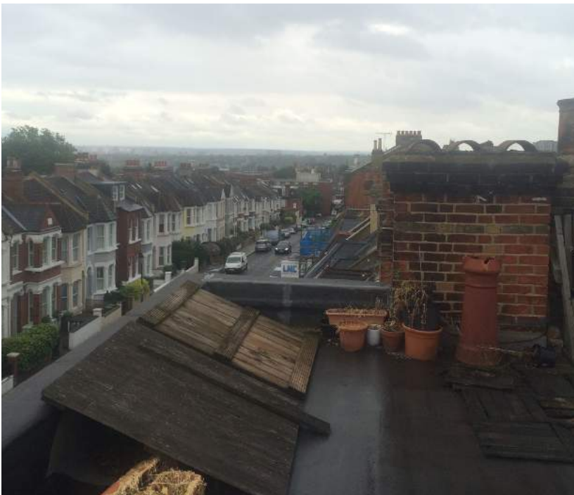
View from the roof looking down Burrard Road towards Fortune Green Road. The roof is in need of major repair works, and shows signs of layers of patching that extend over the parapet and stucco cornice.
