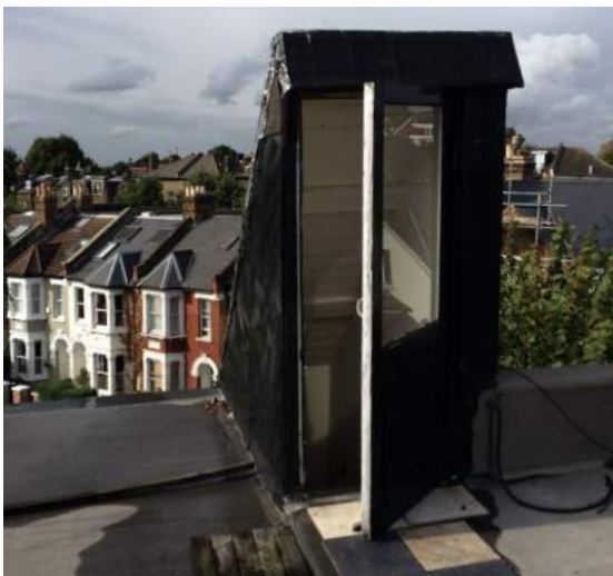
The existing roof access stair housed in a remnant of the original tiled roof volume and brick gable.
