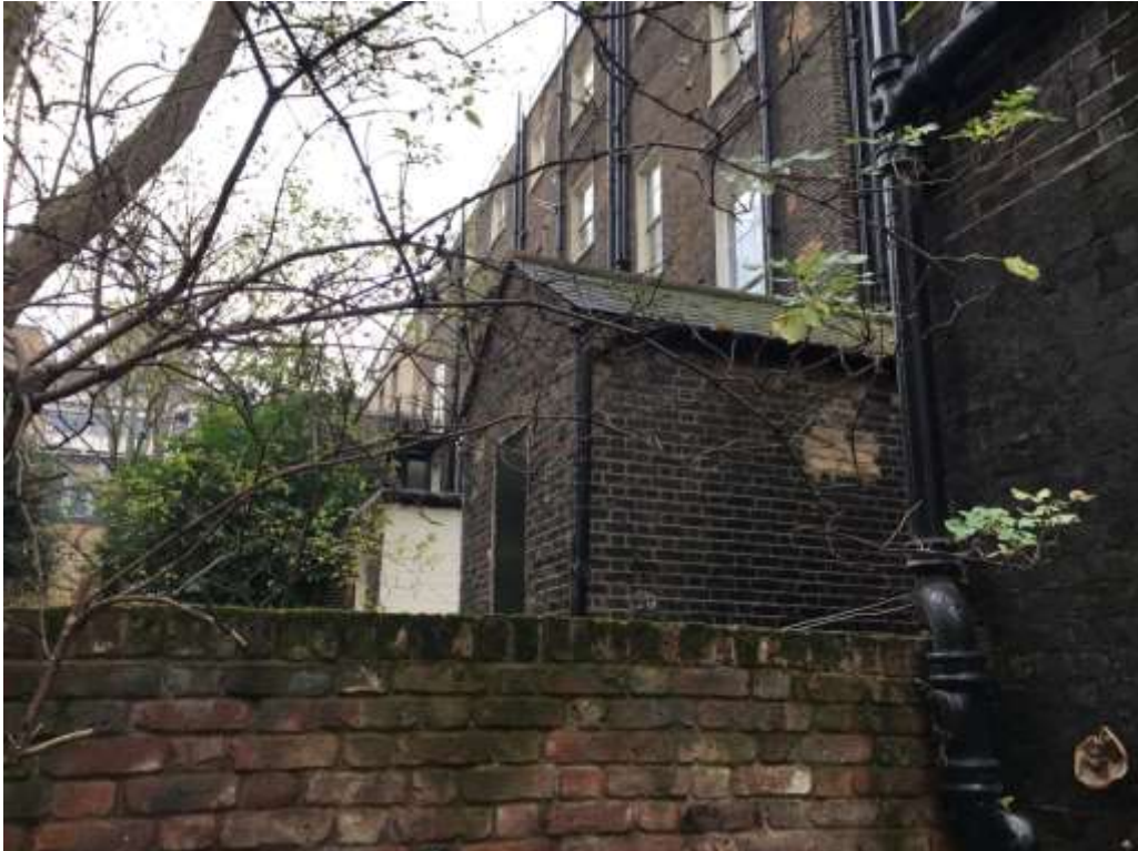
Figure 4.9: Showing the eclectic closet wings to the rear of Nos. 27-32 Torrington Square. On the far right (close quarters) is the three storey closet wing of No. 32. A two storey closet wing can be seen to No. 31 adjoining.
