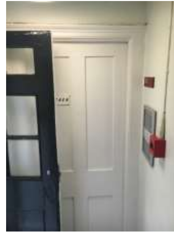
Figure 3.34: 4-panelled door to upper ground floor rear room (centre) and part glazed, part panelled door to garden fire escape (left).
