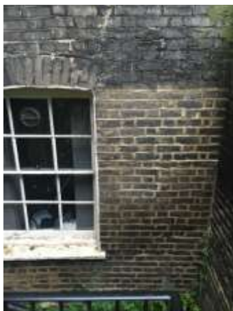
Figure 3.19: Lower ground floor window and low grade brick pointing to northern bay of rear elevation.
