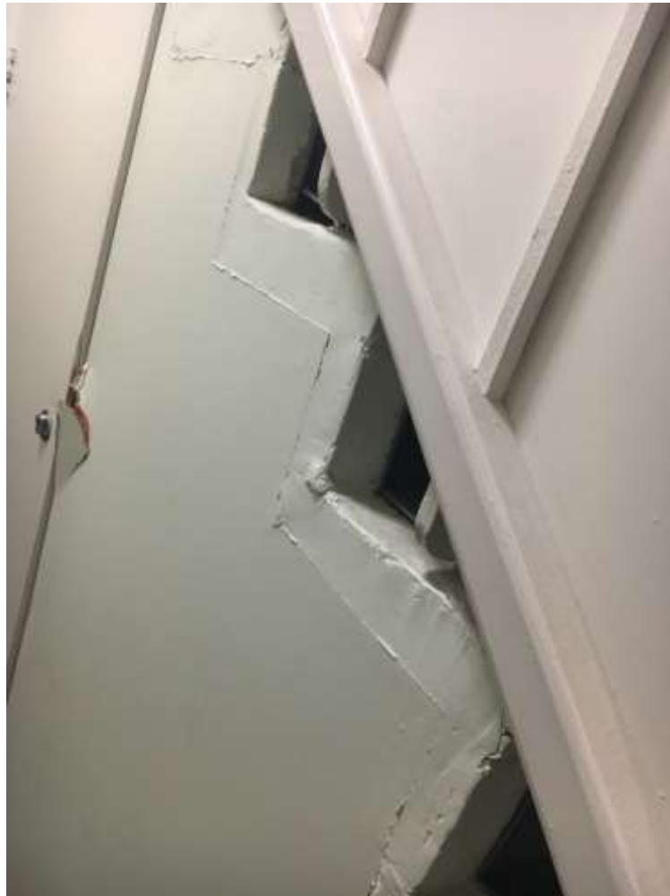
Figure 4.5: Stairs from basement to ground showing original steps and balusters as well as modern cladding
