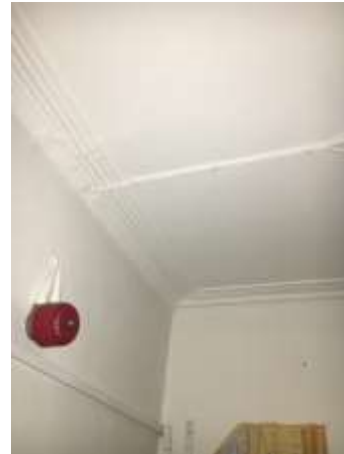
Figure 3.45: Modest later cornicing to rear room.
