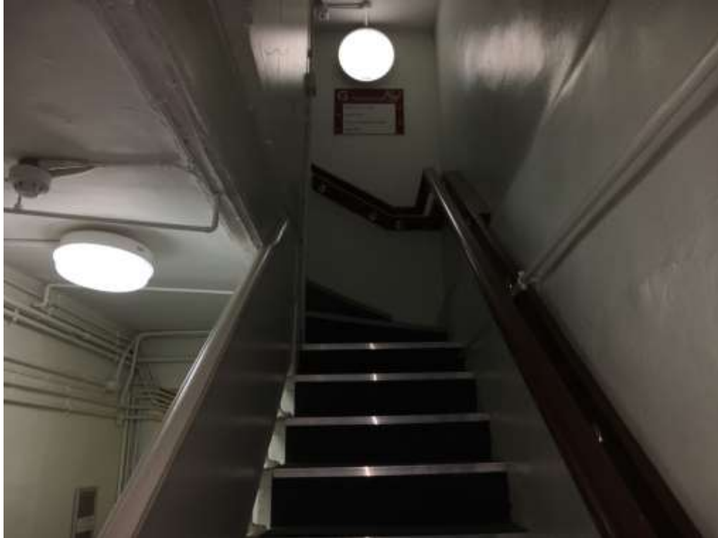
Figure 4.3: Showing existing conduits and cables in the basement hallway
