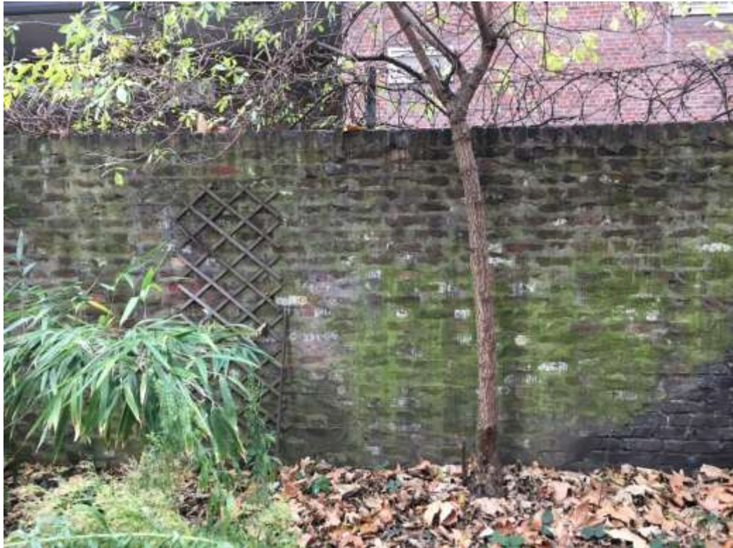
Figure 4.1: Showing the relatively low grade brickwork to the garden boundary wall
