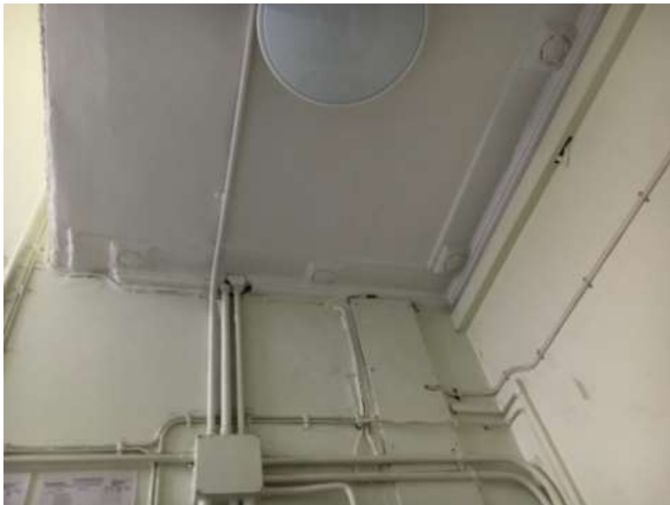
Figure 4.2: Showing existing conduits and cables in the first floor hallway. Historic cornice also visible.
