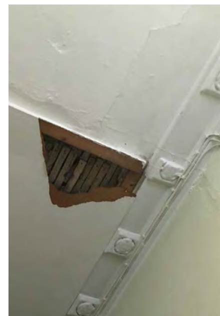
Figure 4.2. Ceiling plaster and moldings to be made good as necessary as per Heritage consultant recommendations
