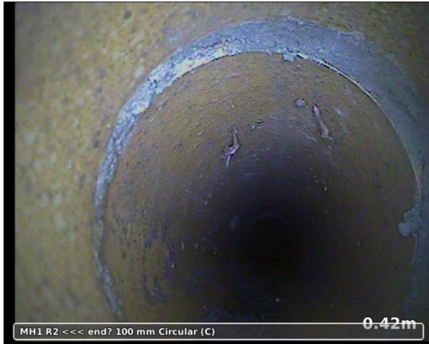
20170516-092920-snap0000.jpg, 00:00:29, 0.42m Joint displaced, medium
