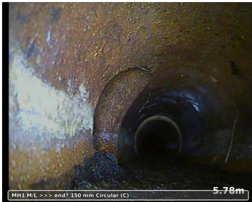
20170516-100118-snap0008.jpg, 00:04:58, 5.74m Crack, circumferential, from 12 to 05 o'clock
