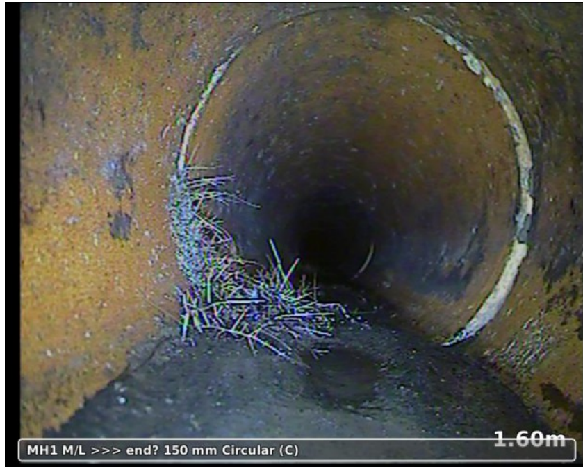
20170516-100118-snap0004.jpg, 00:02:36, 1.60m Settled deposits, hard or compacted, 10 % cross-sectional area loss
