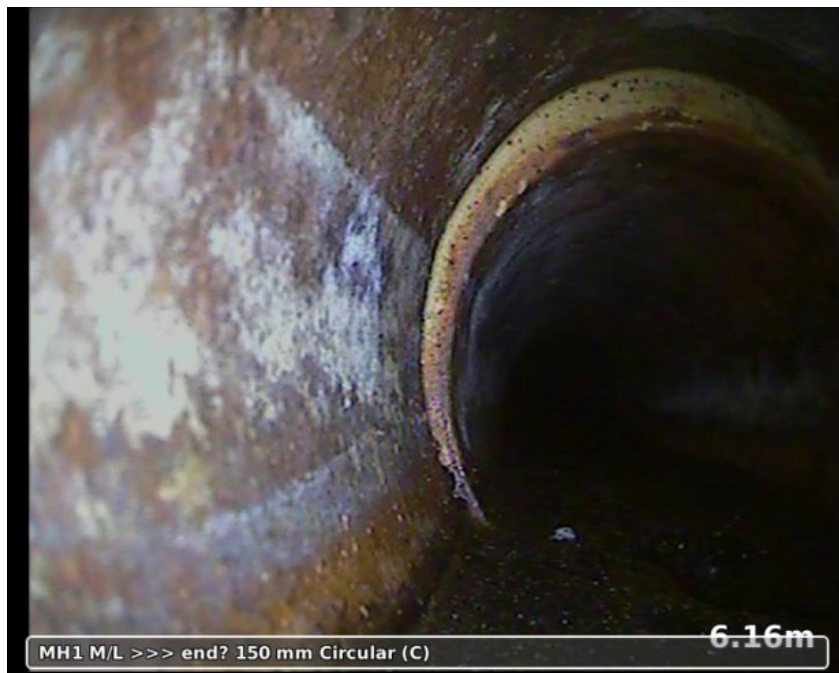
20170516-100118-snap0009.jpg, 00:05:36, 6.16m Joint displaced, medium
