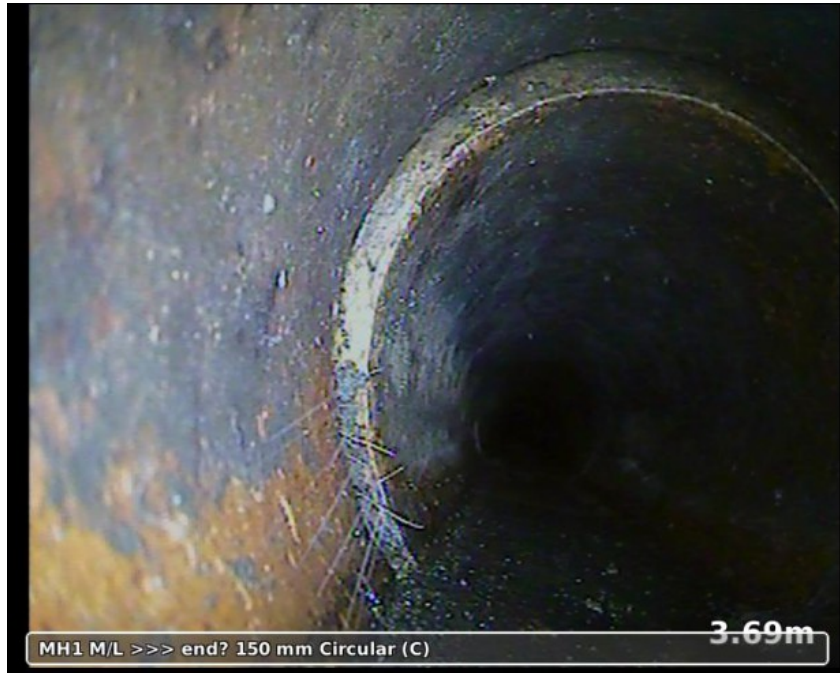
20170516-100118-snap0006.jpg, 00:03:39, 3.69m Joint displaced, medium
