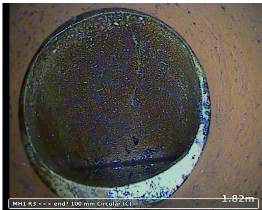
20170516-095202-snap0001.jpg, 00:00:56, 1.82m Joint displaced, medium
