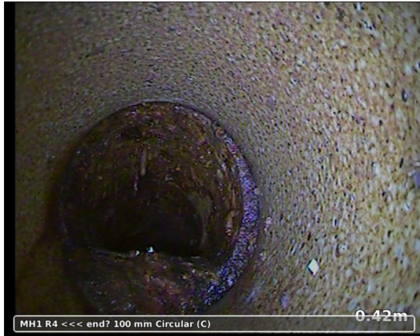
20170516-095512-snap0000.jpg, 00:00:47, 0.42m Settled deposits, hard or compacted, 30 % cross-sectional area loss
