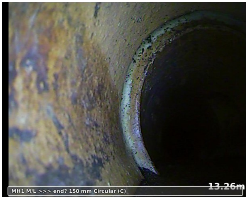
20170516-100118-snap0011.jpg, 00:07:39, 13.26m Joint displaced, medium
