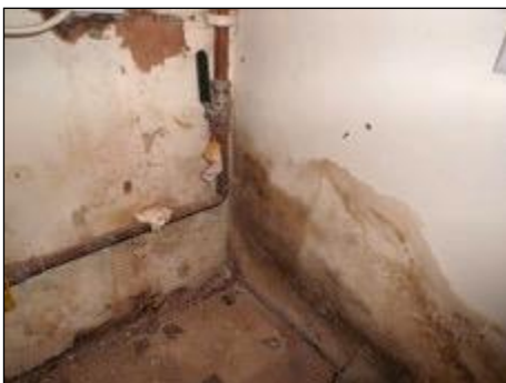
Damp plaster and boarding rear right corner of cellar area
