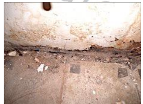
Damp plaster at low level
