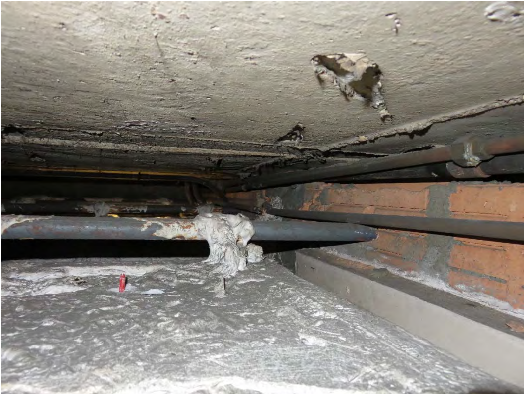
VIEW ABOVE THE LOWER FIBROUS PLASTER CEILING IN THE CORRIDOR OUTSIDE THE KITCHEN
