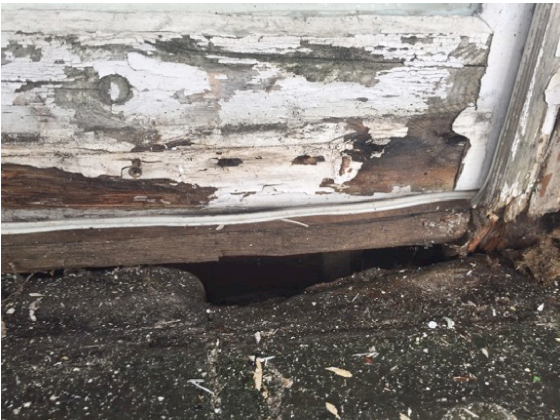
Photograph 2 – Large gap between the balcony and door above indicating lack of cantilever support and deemed an unsafe structure
