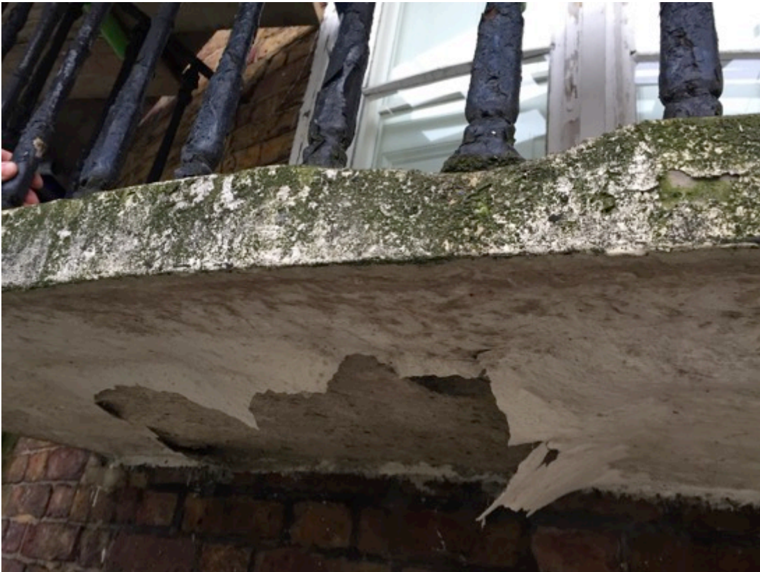
Photograph 1 – Balcony in disrepair
