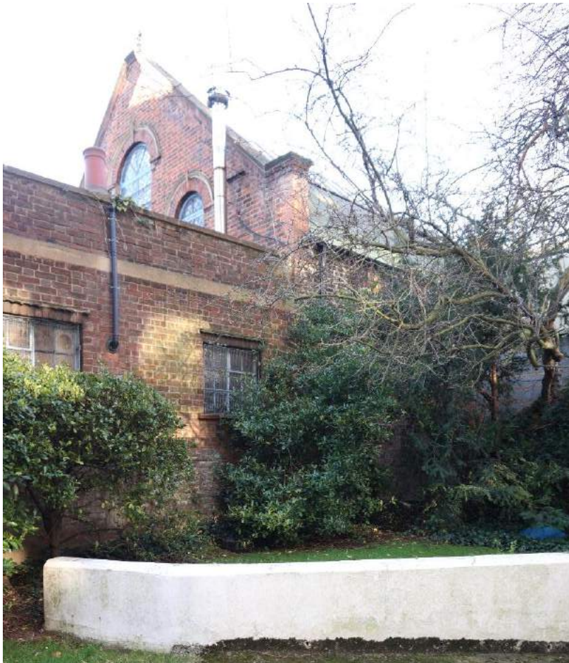
The side elevation of the Temple seen from the access road serving the basement garage in Julian Court
