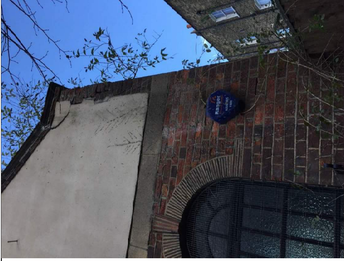
Plate 3: Crack along fascias and brick.
