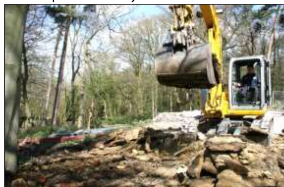
Hard surfacing/structure removal image 2: Machines with a long reach can be used to lift out heavy surfacing and structures as long as the machine sits outside the RPA and the exposed surface is protected before there is any further access.
