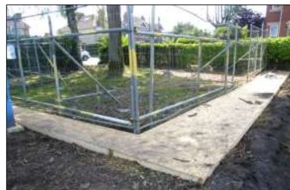
Ground protection image 2: Plywood fixed to a wood frame is another effective method of protecting soil from pedestrian compaction.
