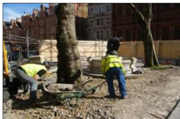
Hard surfacing/structure removal image 4: These trees had impermeable surfacing right up to their trunks, which had to be removed by hand before installing new structures.
