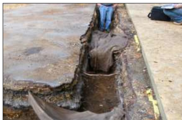
Excavation image 4: Exposed roots must be protected from light, drying out and extremes of temperature by covering with hessian sacking and boards until they can be covered back with soil.
