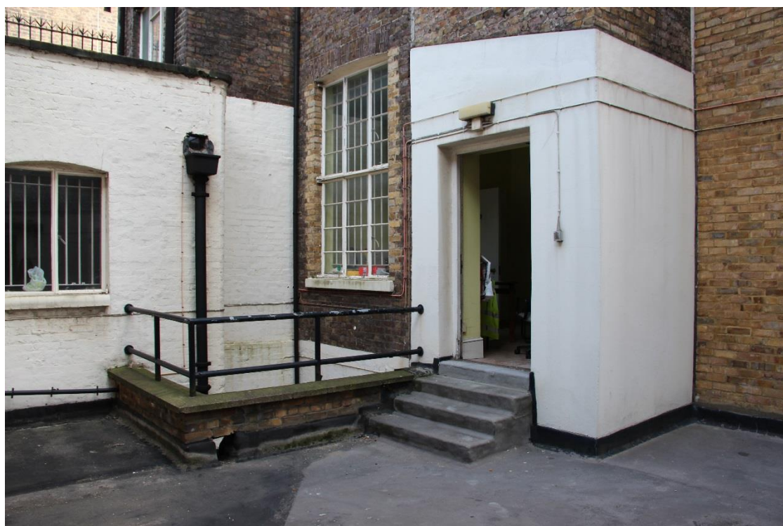
1 Montague Street - Rear – Side Elevation Existing light fittings and cabling to be removed. New railing added to existing parapet. Height provided to comply with current building regulations.
