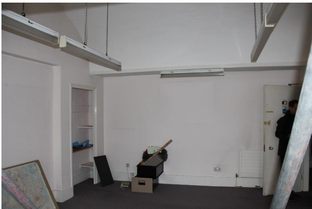
Existing lighting to be removed and replaced. Refer to drawing (35)AP005. Ceiling to be repaired and made good following works.
