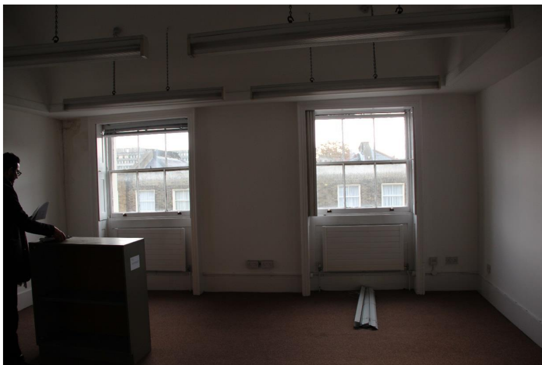
Windows to undergo full overhaul to ensure good working condition and receive full redecoration.
