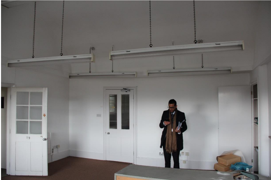
Existing lighting to be removed and replaced. Refer to drawing (35)AP004. Ceiling to be repaired and made good following works.
