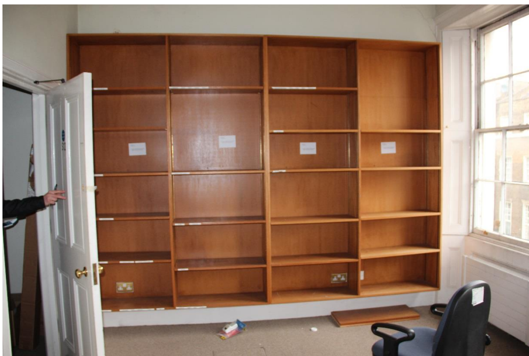
Existing room 1AMS/4/012: Walls to be made good where necessary following removal of existing wall adjoining room 1AMS/4/014. Existing windows and shutters to undergo full overhaul to ensure good working condition and receive full redecoration
