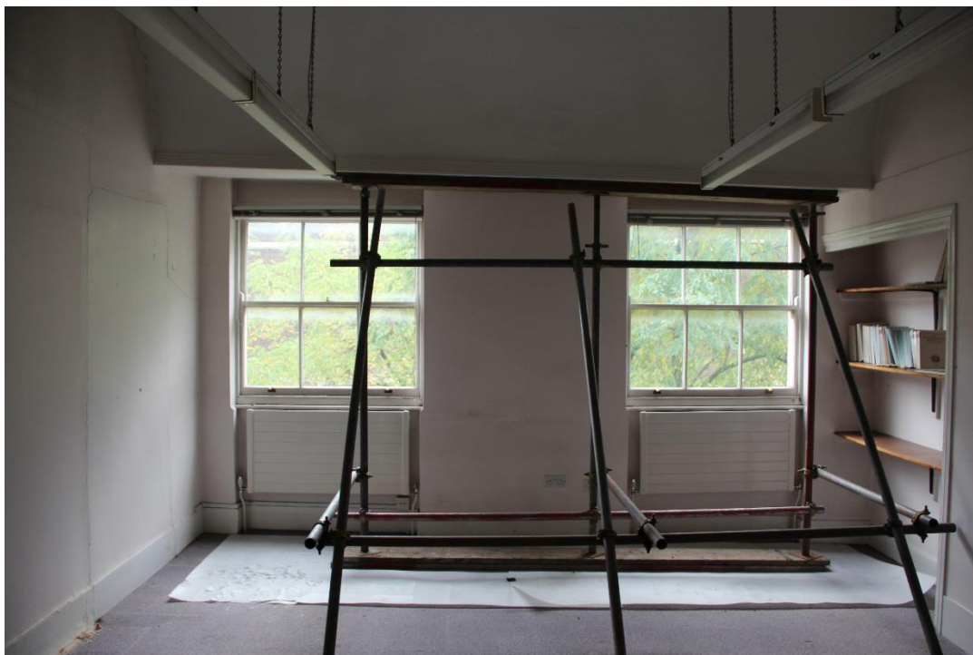
Windows to undergo full overhaul to ensure good working condition and receive full redecoration. Redecoration throughout;
