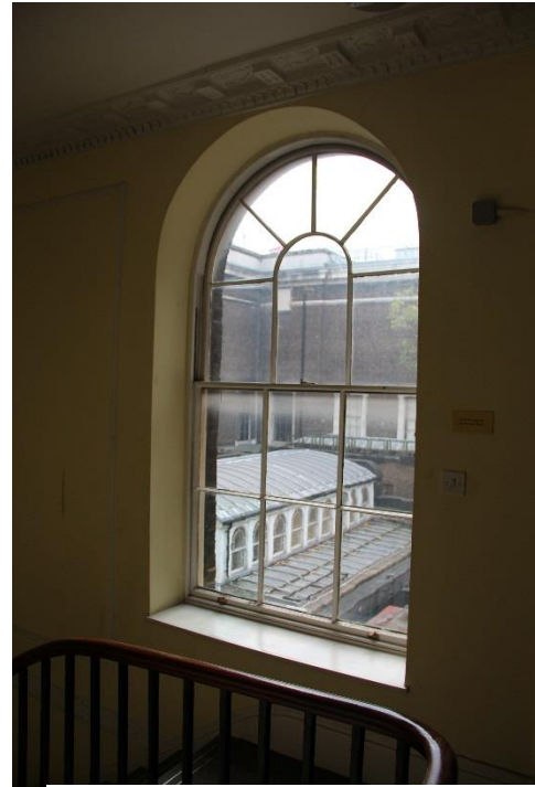
Window to undergo full overhaul to ensure good working condition and receive full redecoration.
