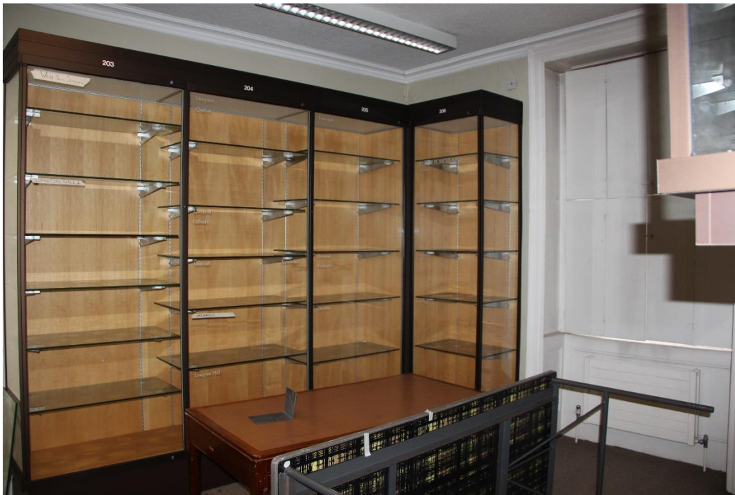
Metal work and damaged modern plaster finishes following removal of museum shelving, to be carefully removed and replaced with lath and plaster/original plaster to match existing adjacent. Redecoration throughout.
