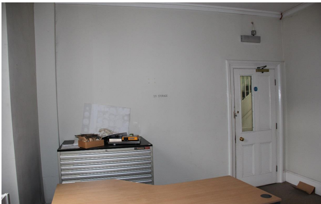
To be confirmed on site if wall provides 30 min fire resistance. If it doesn't, wall to be overboarded with new fire resistant board to provide the required 30 minute fire protection. Cornice carefully removed and set aside with care. Reinstated and redecorated when the overboarding of the wall is completed. If damage occurs refer to method of statement. If it does, damaged plasterboard replaced with plasterboard to match existing adjacent. Redecoration throughout. Existing door opening infilled with 30 minure fire resistance partition.
