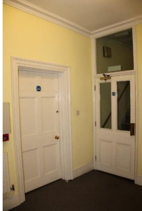
Existing doors to be upgraded for fire protection and redecorated. Refer to door schedule.
