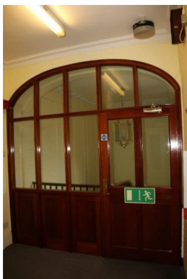
Existing mahogany door and glazed panel to be removed to reinstate original condition
