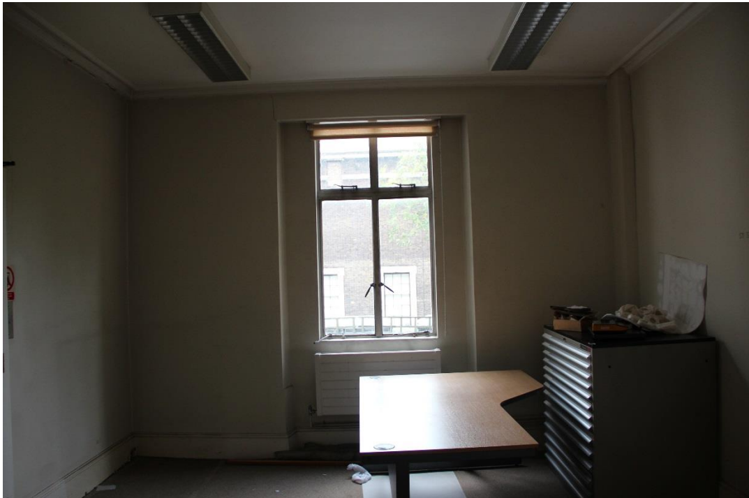
New suspended ceiling to be installed to conceal services in specific area of room. See BDP drawing (35)AP004
