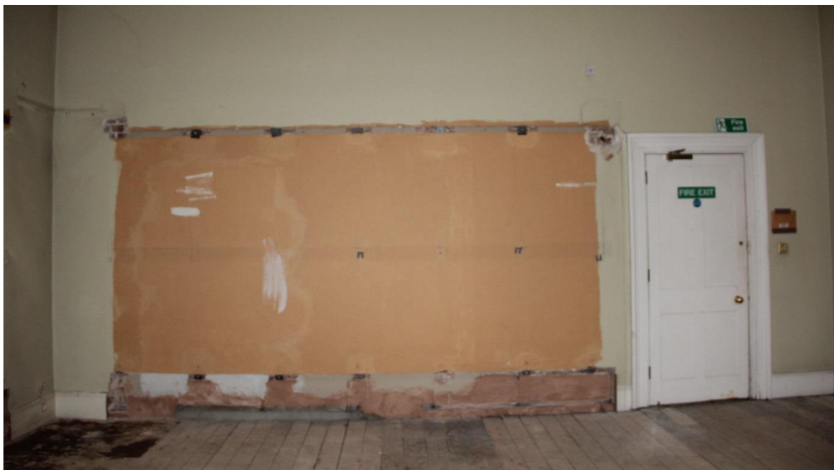
ELEVATION 4 - Metal work and damaged modern plaster finishes to be carefully removed and replaced with original plaster to match existing adjacent. Redecoration throughout. Existing door containing asbestos to be replaced with new FD30 door.
