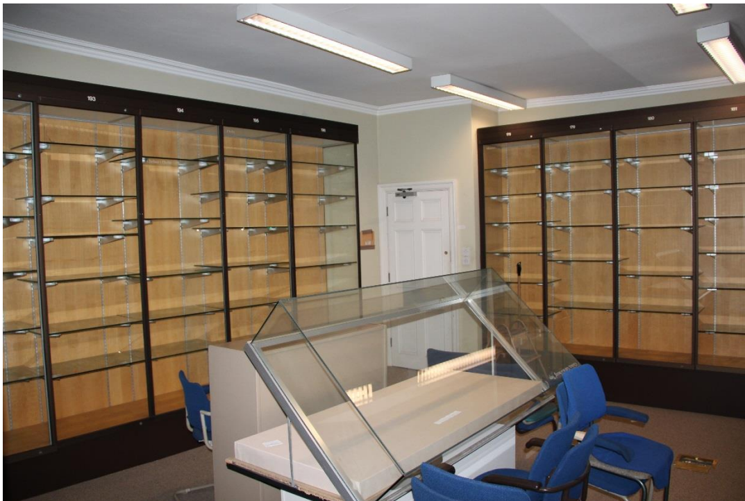
Metal work and damaged modern plaster finishes following removal of museum shelving, to be carefully removed and replaced with lath and plaster/original plaster to match existing adjacent. Redecoration throughout. Existing door refurbished and redecorated. Fire upgrade required. Refer to (67)AP004. Ironmongery to be retained and refurbished.
