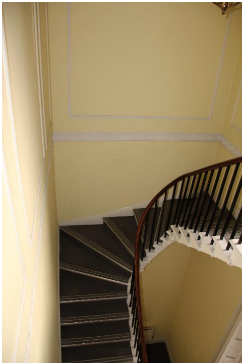
Stairs, balustrade and handrail to be fully refurbished and redecorated
