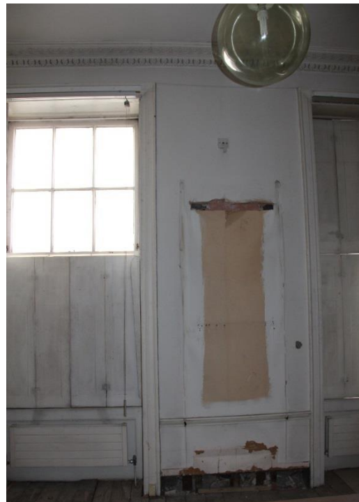
ELEVATION 2 - Existing radiators to be carefully removed with all other existing services. Original timber panelling to front elevation to be retained, refurbished and redecorated. Windows to undergo full overhaul to ensure good working condition and receive full redecoration.
