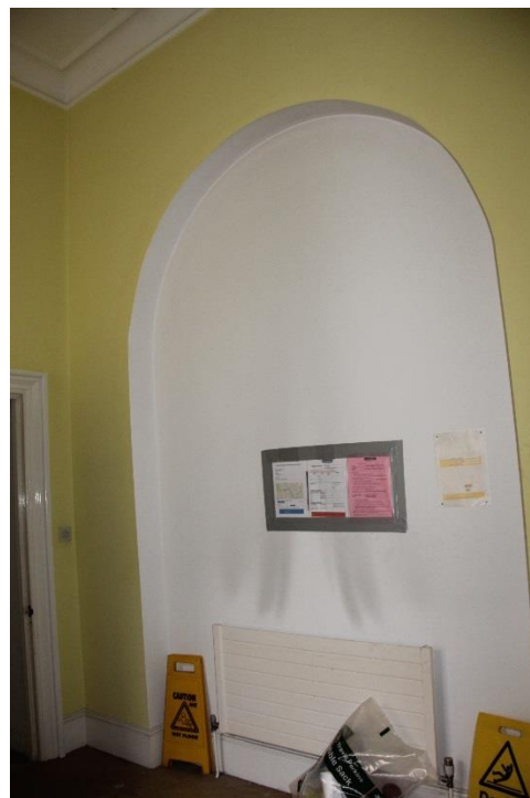
ELEVATION 6 – Modern timber stud and plasterboard infill to be carefully removed to reinstate original opening
