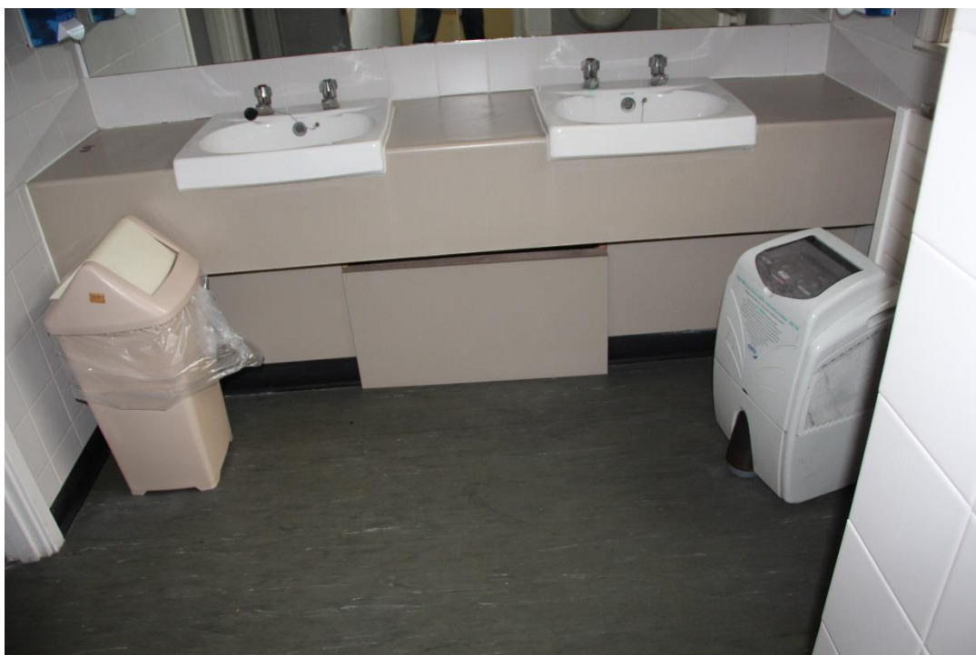
Existing sanitary ware to be carefully removed. New plasterboard stud partitions to be formed to create kitchenette. Damaged areas of wall to be repaired. Redecoration throughout.
