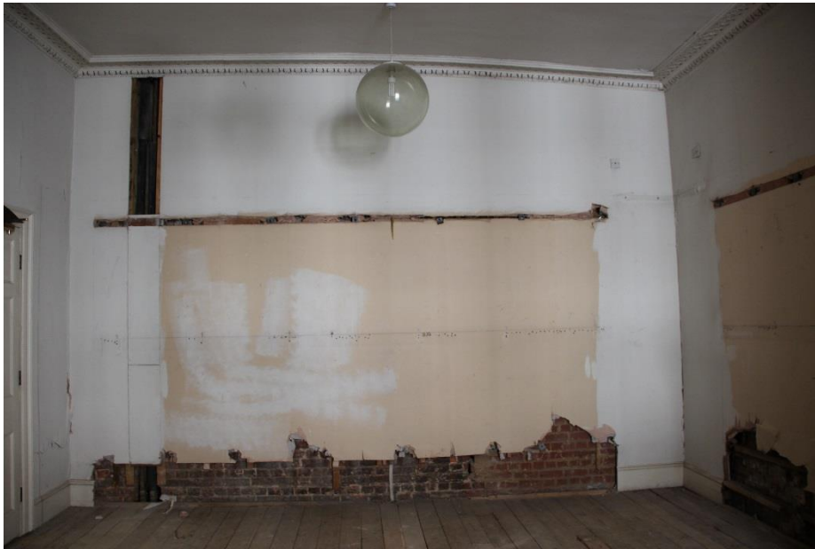
ELEVATION 3 - Load Bearing masonry partition with existing service riser incorporated. Existing services to be removed. Metal work and damaged modern plaster finishes to be carefully removed and replaced with lath and plaster to match existing adjacent. Redecoration throughout.
