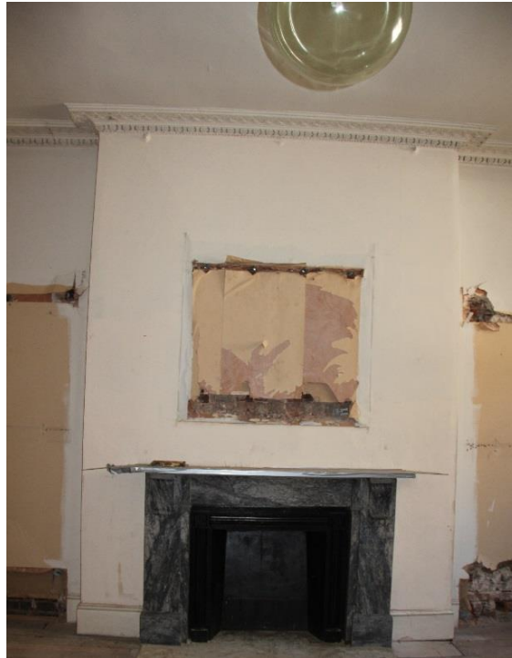
ELEVATION 1 - Fireplaces to be protected and retained. Non-abrasive cleaning required. Sections of modern replacement wall finishes to be carefully removed and replaced with lath and plaster to match existing adjacent.
