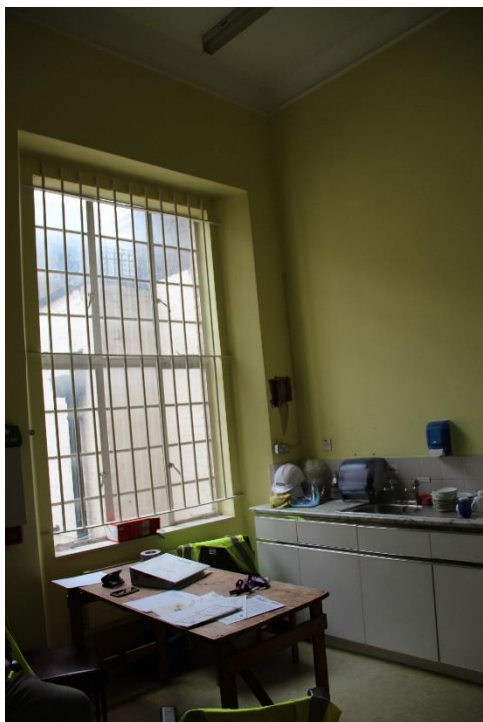
ELEVATION 5 - New sash window 1A-G-W03 to replace existing rear window. Refer to BDP drawing (31)AD002
