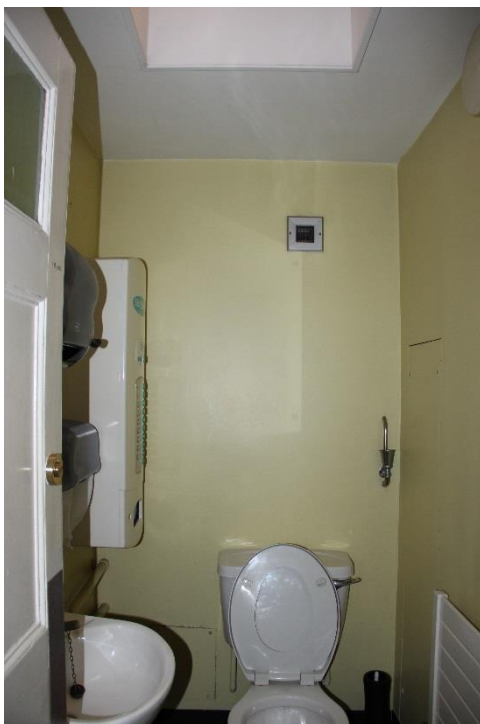
Existing sanitary ware to be carefully removed. Damaged areas of wall to be repaired and new sanitary ware to be fitted. Redecoration throughout.
