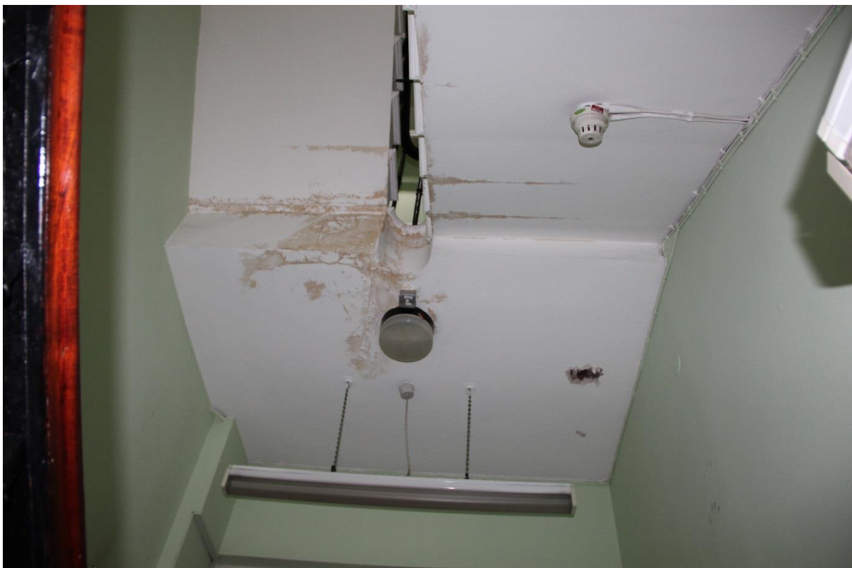
Where evidence of dampness exists, assess condition and associated structure, rectify source and carry out repairs and relining where necessary;
