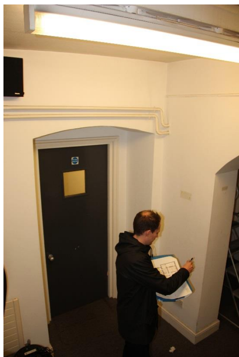
Existing walls, ceiling, doors to be retained, architrave and skirting to be redecorated
