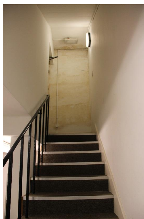
Evidence of dampness to be assessed and repairs to be carried out accordingly
