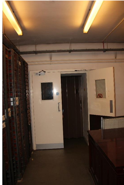
New walk-on floor grille to be installed within existing lift shaft to access services and doors to be replaced
