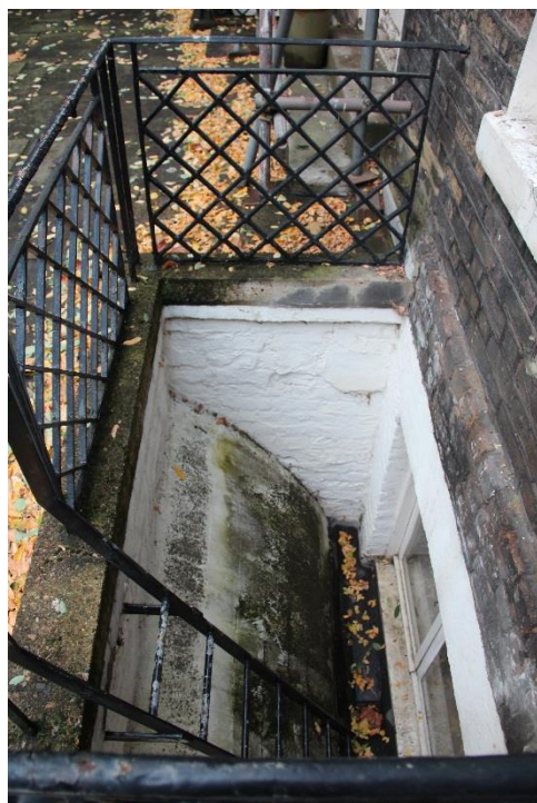
Existing light wells and balustrades to be cleaned and redecorated
