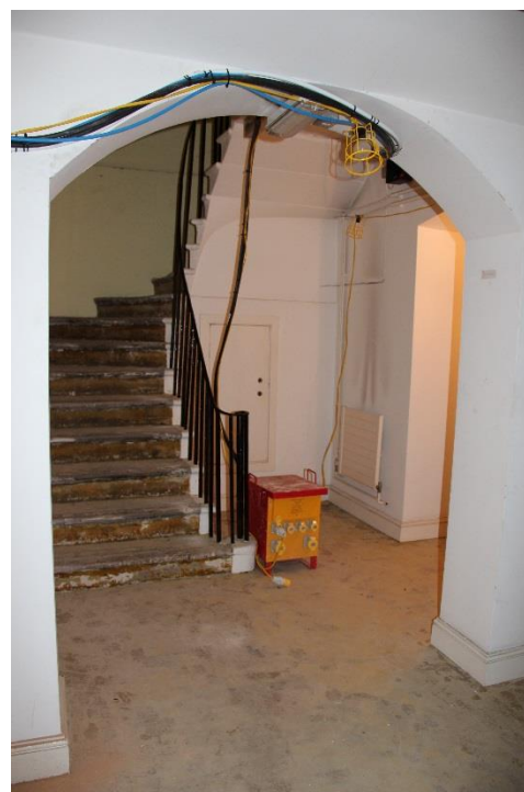
New fire resistant door 1-LG-D16 to be fitted in existing arched wall opening, Refer to detail (32)AD002
