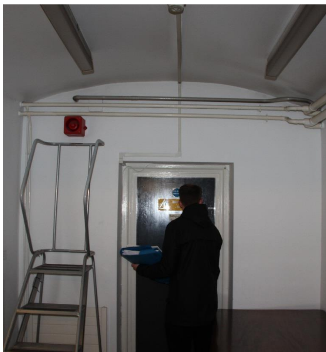
New ceiling bulkheads required to run each side of the ceiling to contain incoming services. See BDP drawing (50)AD102
