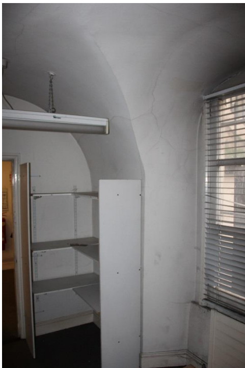
Existing internal door, architrave, skirting, window, walls and ceiling to be redecorated
