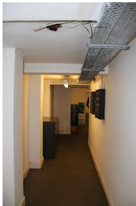
New entrance door to be fitted and two new openings to be made in existing wall to accommodate toilets and shower
