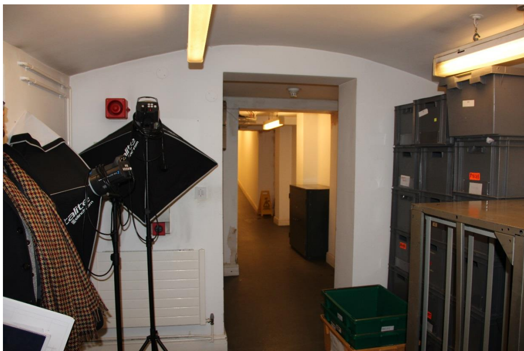
New door and partition to be fitted in existing passage to create entrance to the proposed toilets
