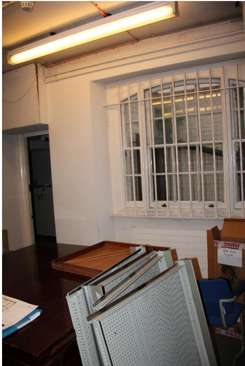
Existing door to 1AMS/1/004 to be removed and opening to be infilled.
