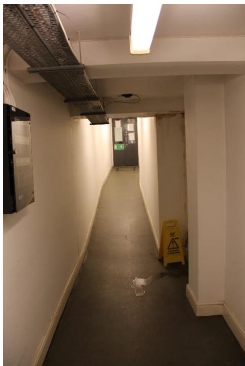
Access to existing tunnel to be blocked up to form toilet and shower area
