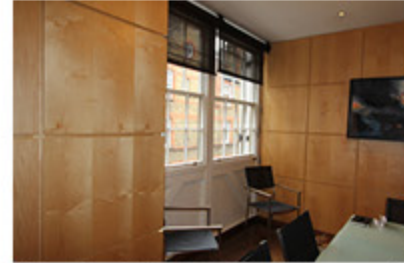
Joinery from the 1990s in the sitting room next to the kitchen on the first floor.
