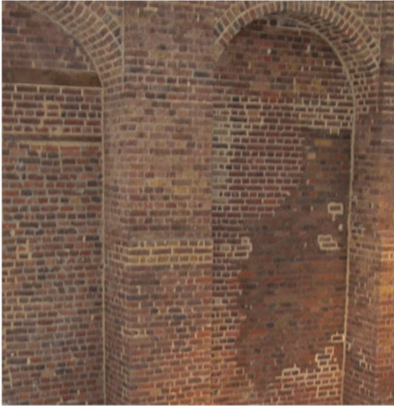
North Main Hall showing imperfections in the brickwork patterns, possibly due to past damage.
