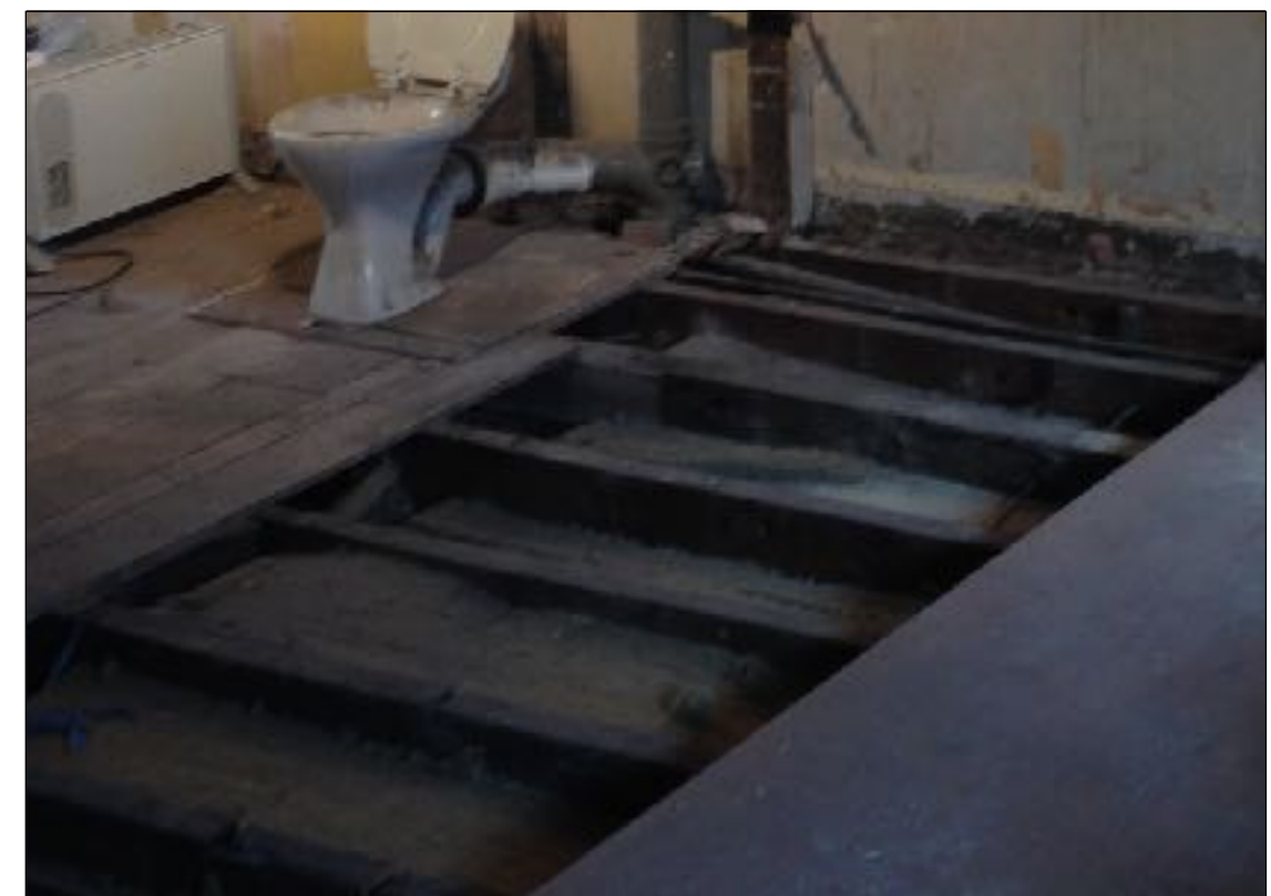
Above : Deviation of floor joists
