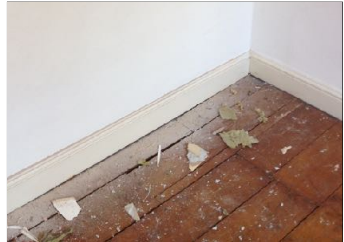
Above : No apparent board nailing and evidence of cut and splice work
