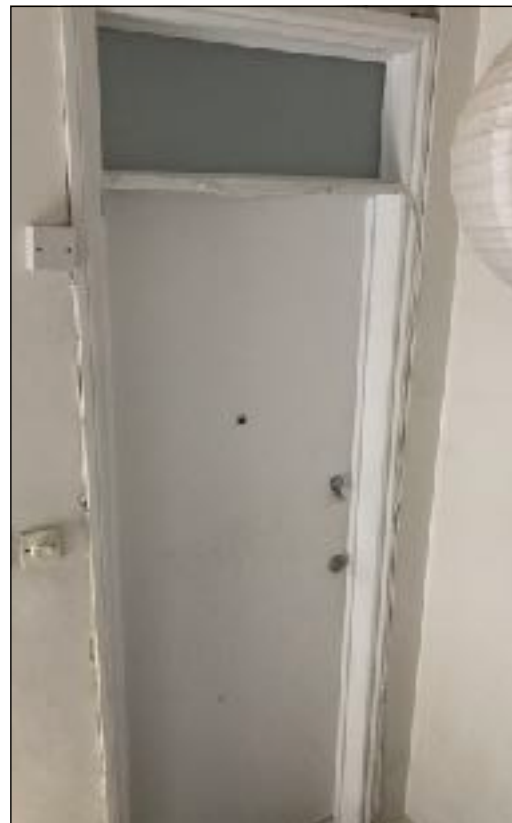
Above: Entrance door to the apartment was replaced with like-for-like door (architrave not replaced)
